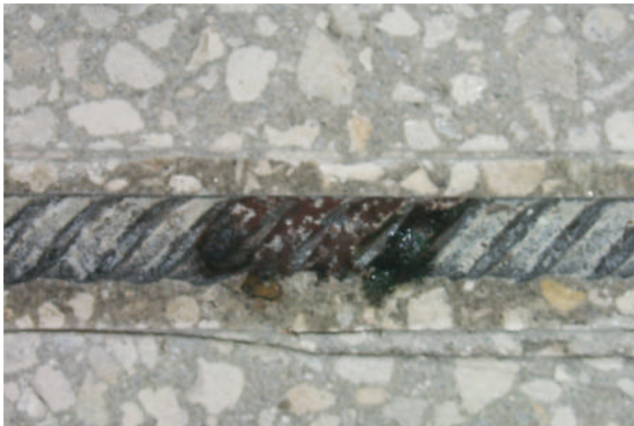
Figure 31: Photograph of the locally corroded region on the exposed top half of the upper rebar of Specimen 10 (HA0.41) after sectioning.
