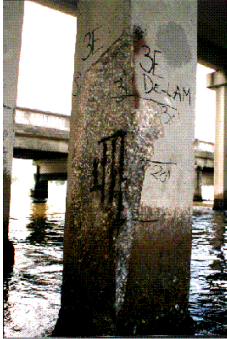
Figure 2: Photograph of a cracked and spalled marine bridge piling.
