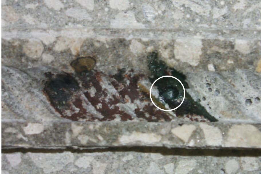
Figure 32 Close-up view of the rebar trace in the concrete at the corrosion site of Specimen 10 (HA0.41).
