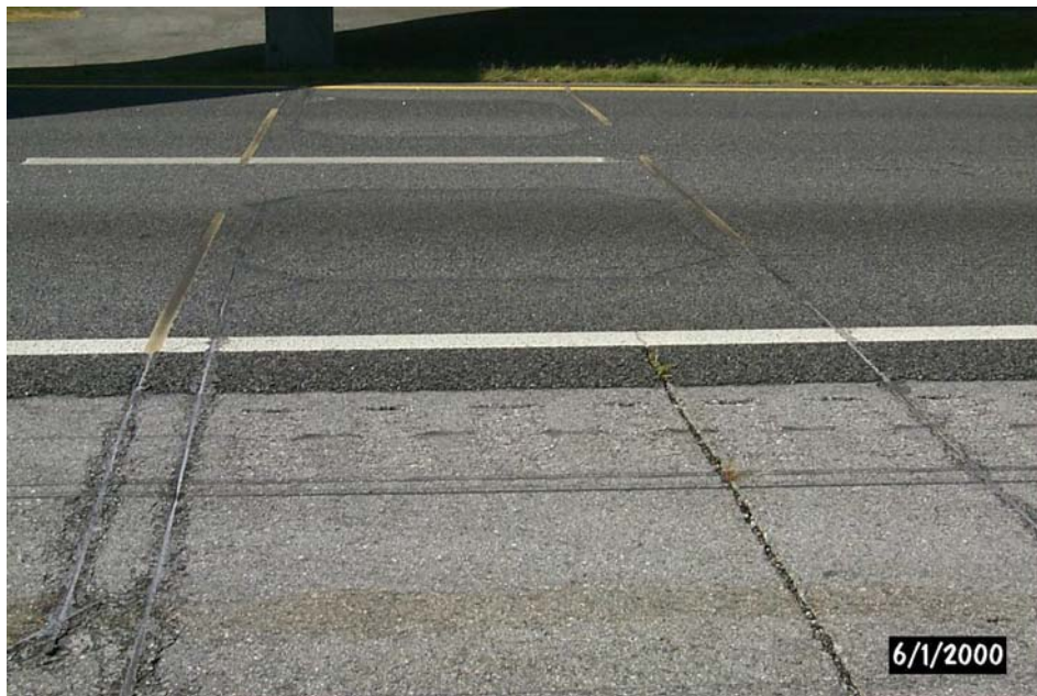
FIGURE 1-1. Piezoelectric Axle Sensor Installed at TTMS # 9936
