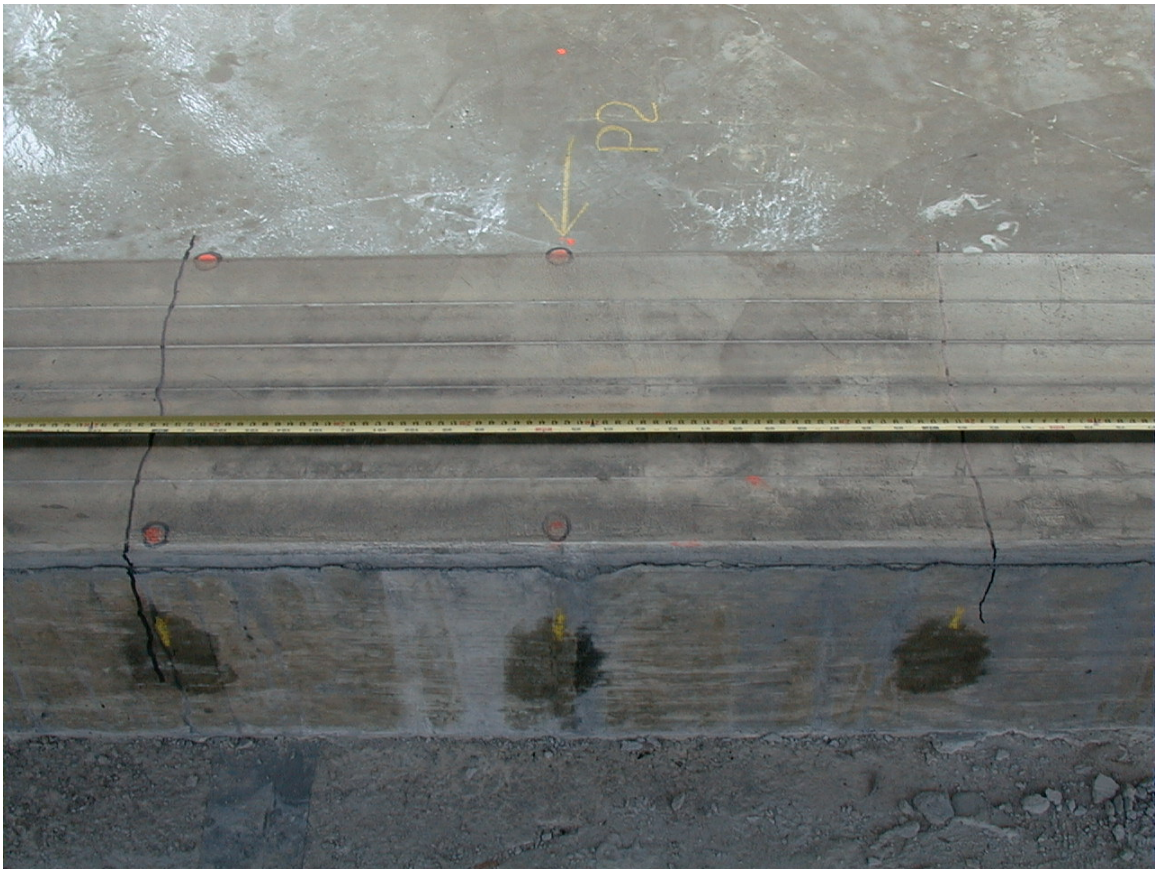
Figure 50. Transverse cracks at mid-edge of Slab 2C
