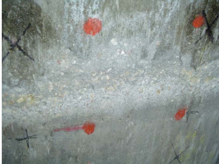
Figure 4.8: Surface scaling due to sulfate crystallization.
