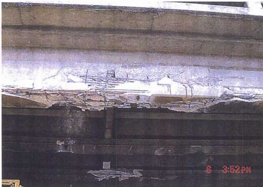
Figure 1-4: Close-up of Damage on the West Fascia Girder in the Vicinity of the Diaphragm
