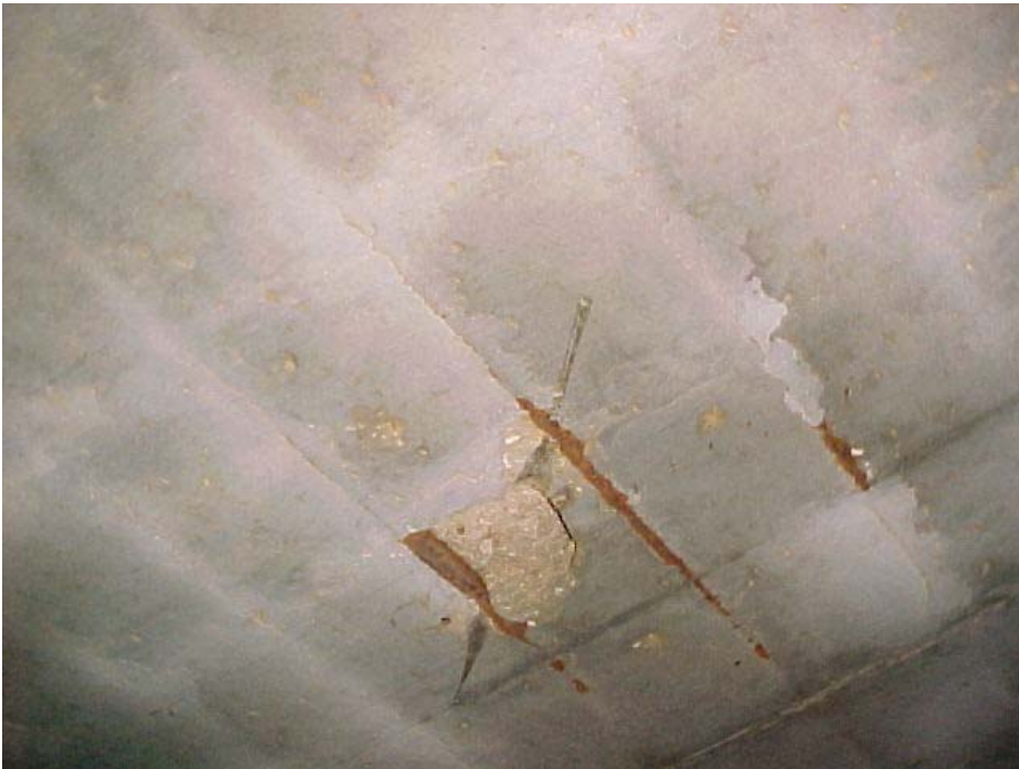
Figure 3.5: Exposed and Corroded Reinforcing Steel
