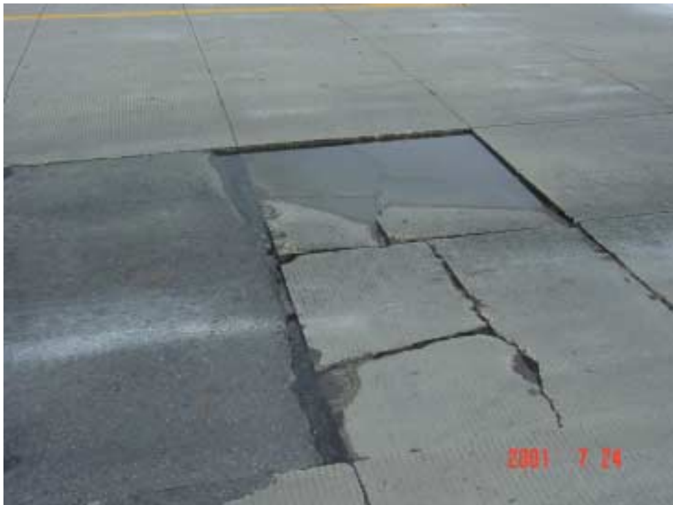
Figure 3.17 AC Patches and Cracked Panels at the Beginning of Section S4E
