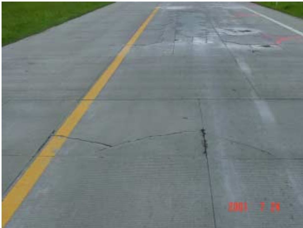
Figure 3.21 Cracked Panels at the End of Section S5E
