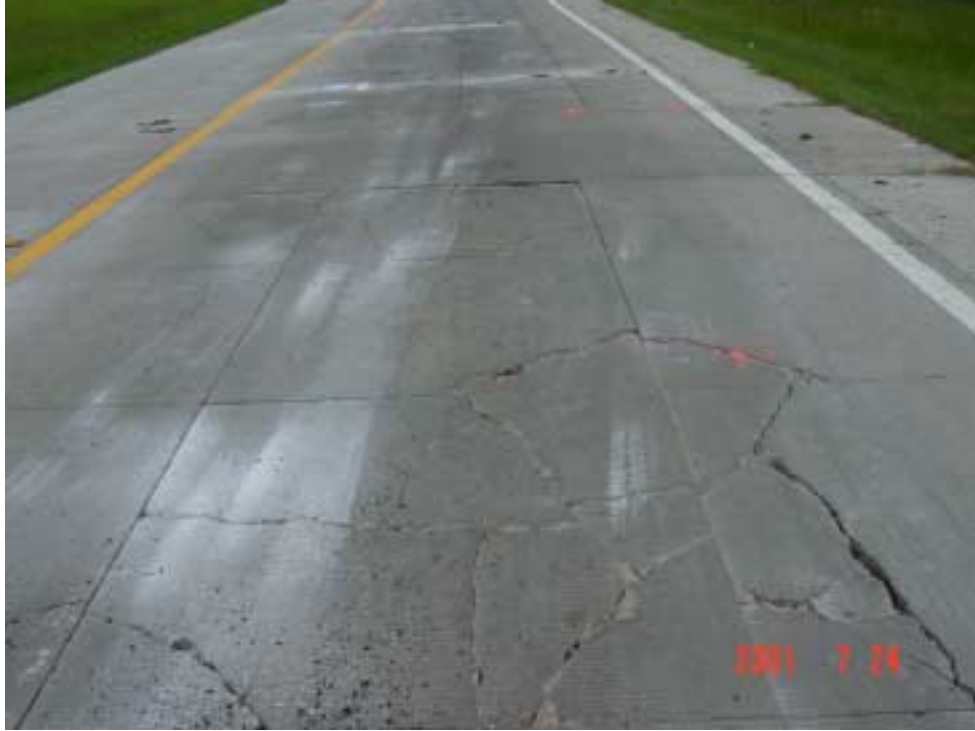
Figure 3.10 Cracked UTW Panels at the End of Section S2W
