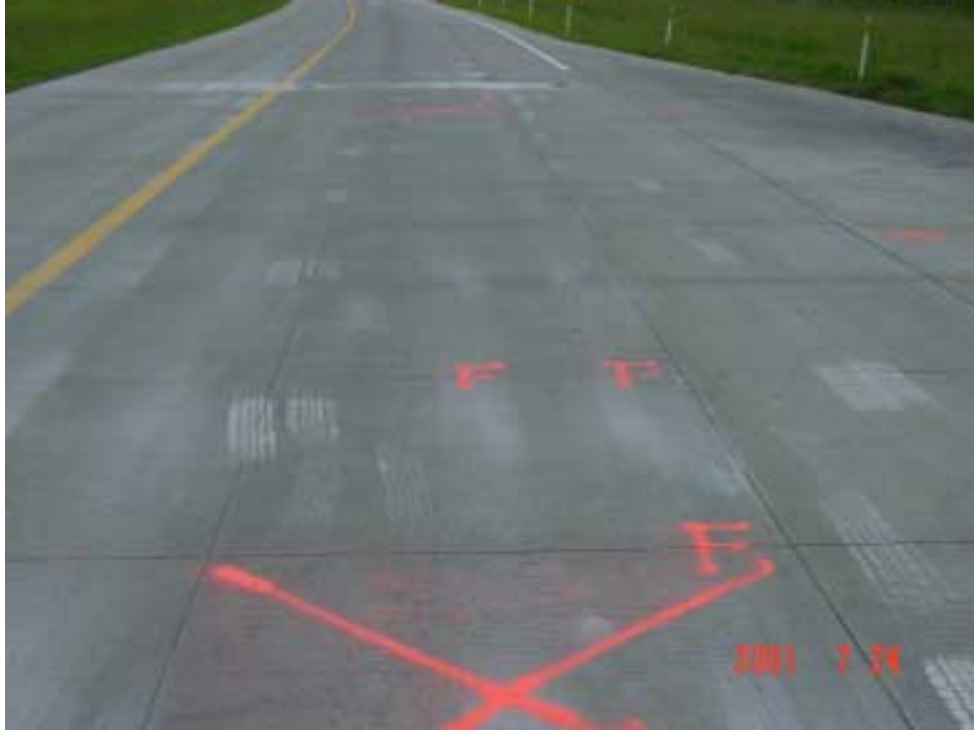
Figure 3.20 Close-up of Panel B30 of Test Section S5E
