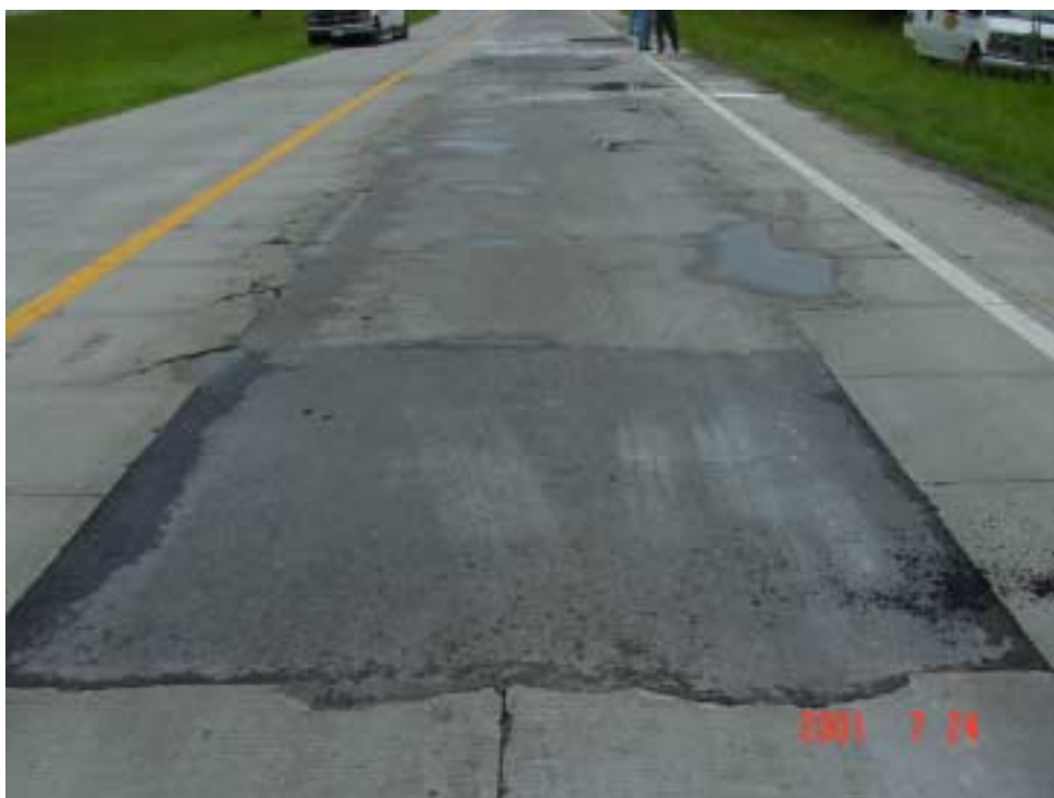
Figure 3.6 Asphalt Patch, B31 and C31 of Test Section S1W
