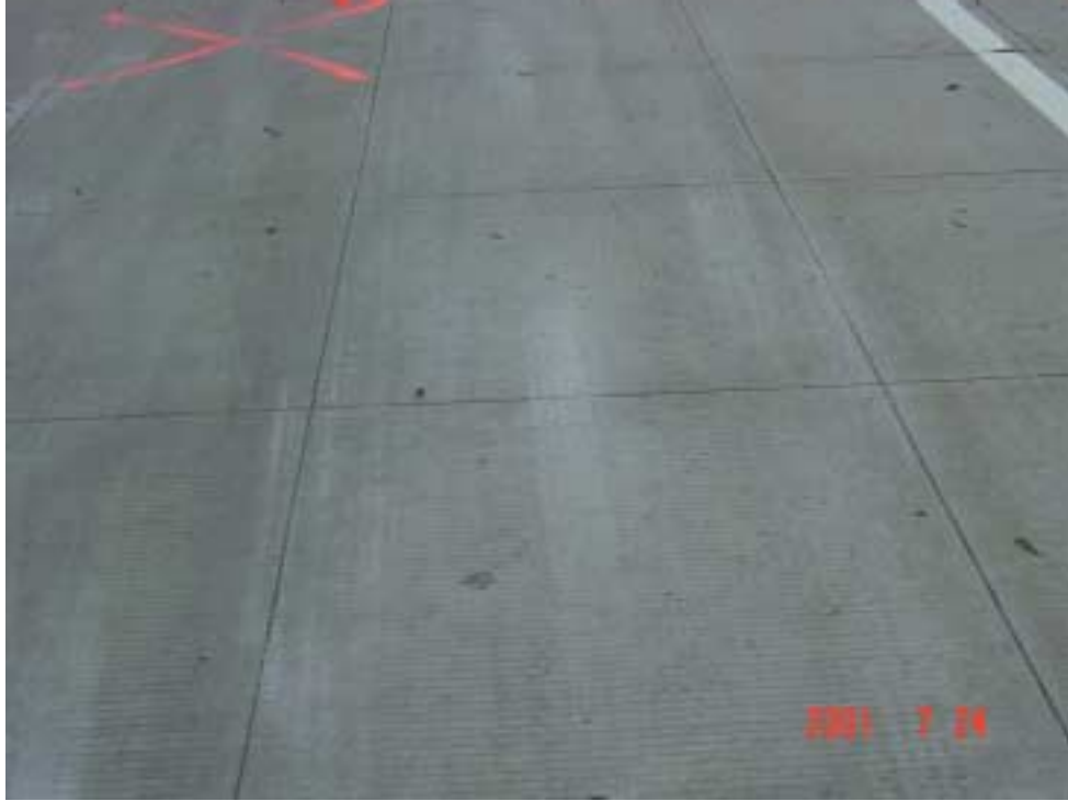
Figure 3.16 Close-up of Panel C36 of Test Section S4E
