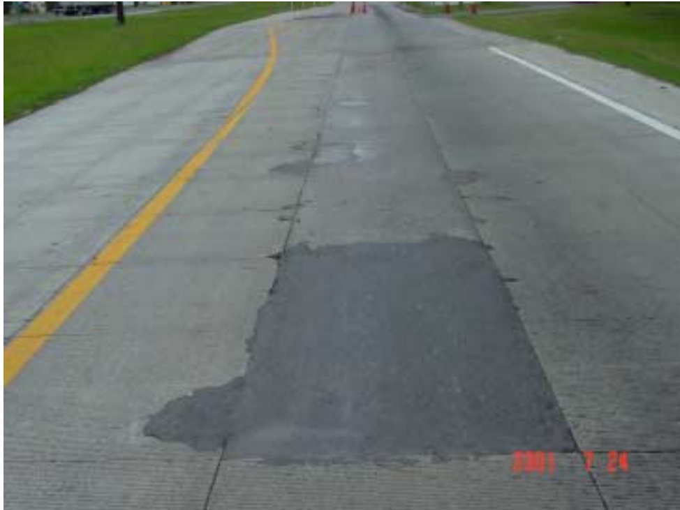
Figure 3.14 AC Patch on Panels B at the end of Section S3W
