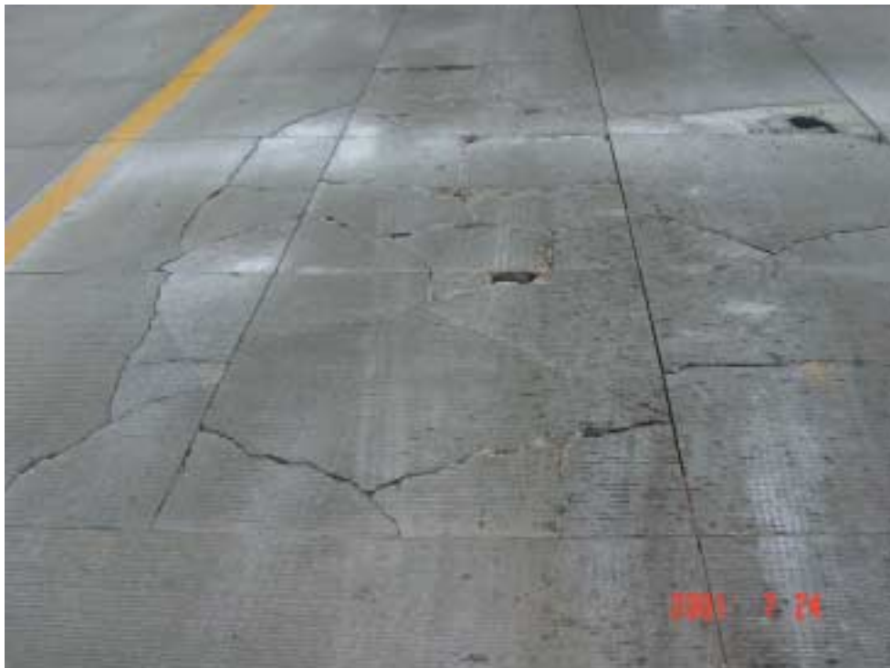
Figure 3.13 Shattered Slabs at the Beginning of Section S3W
