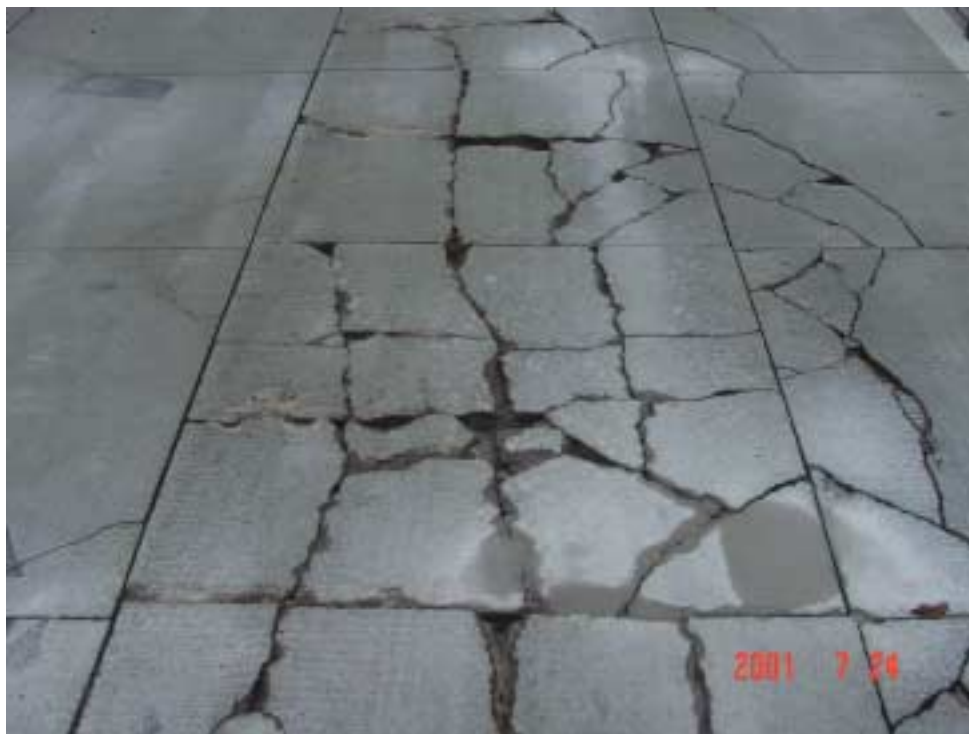
Figure 3.5 Shattered Panels, C15 of Test Section S1W
