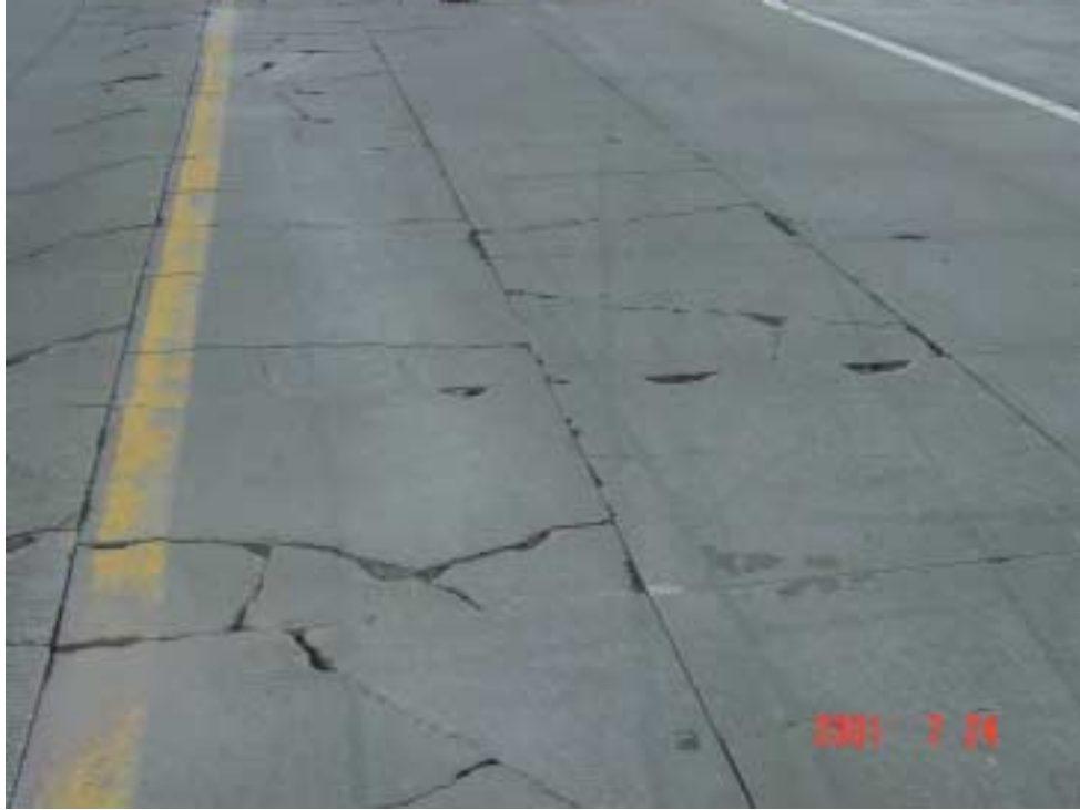
Figure 3.18 Shattered Panels at the End of Section S4E
