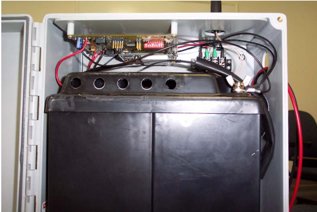
Figure 3. The RMU electronics is shown, along with the Enser batteries and the terminal block used to connect the cathodic protection application cabling.
