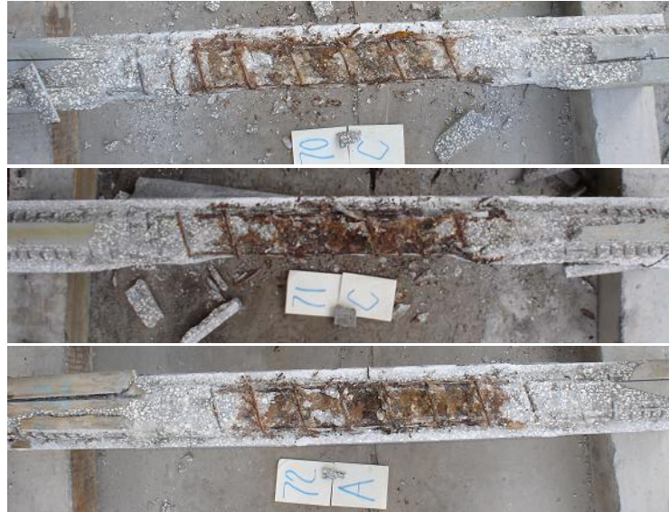
Figure 7.46 Distribution of Corrosion Product in #70 (T), #71 (M) and #72 (B)
