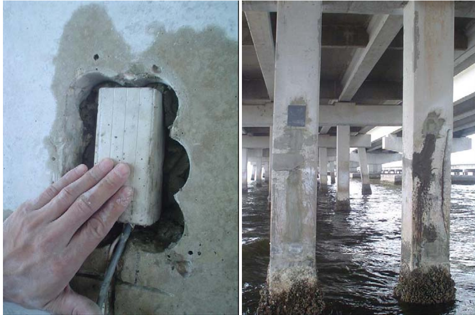
Figure 10.13 Commercial Probe Installation
