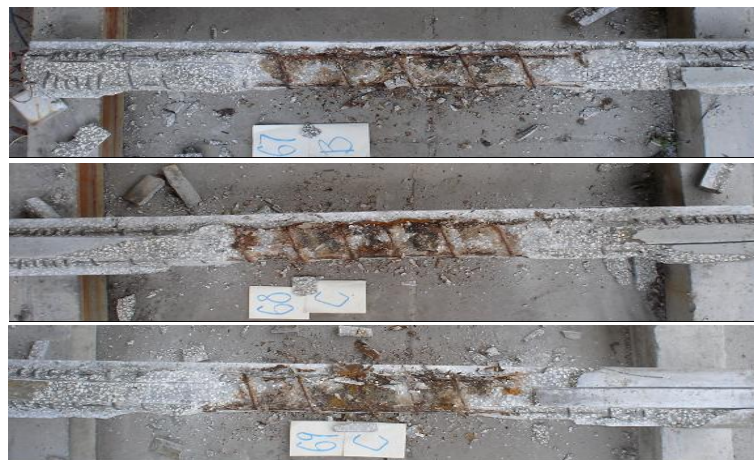
Figure 7.44 Distribution of Corrosion Product in #67 (T), #68 (M) and #69 (B)
