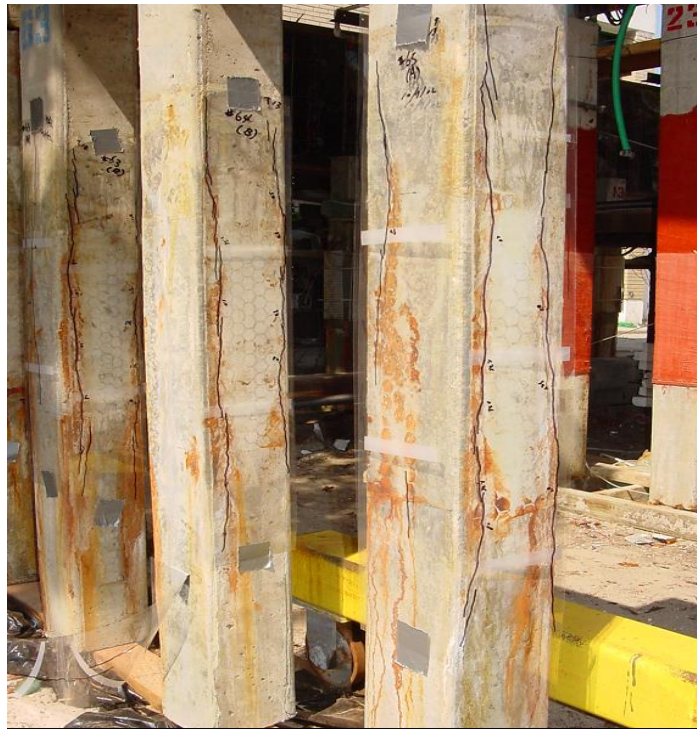
Figure 7.3 Crack Survey after 125 days
