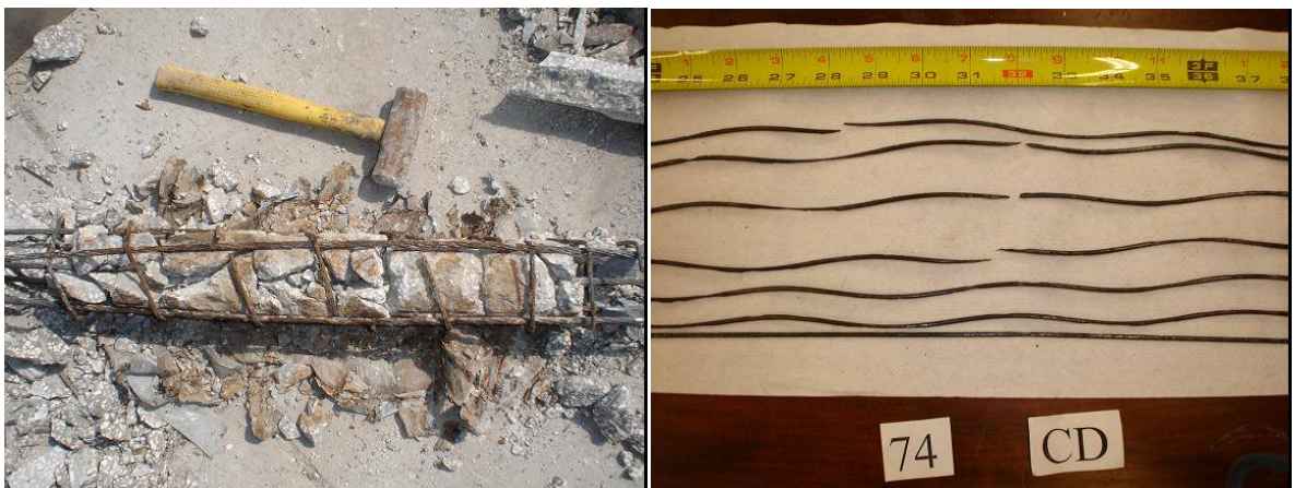
Figure 7.37 Retrieved Steel Cage and Disassembled Wires
