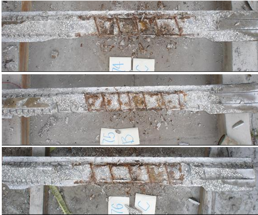
Figure 7.48 Distribution of Corrosion Product in #74 (T), #75 (M) and #76 (B)
