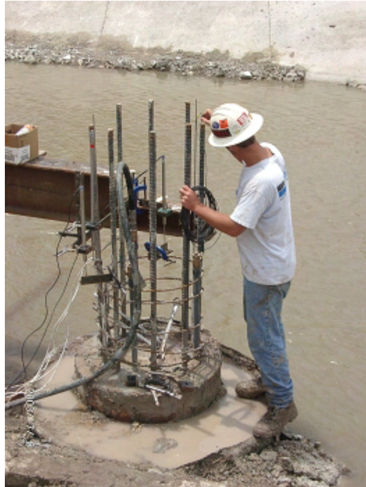
Figure 4-156 FM 507: Instrumentation setup on the west shaft.
