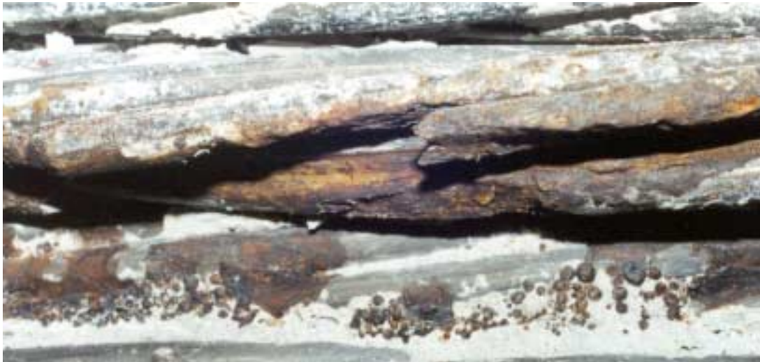
Figure 7. Broken wire in one of the strands of Tendon #2 of Span 40-A.
