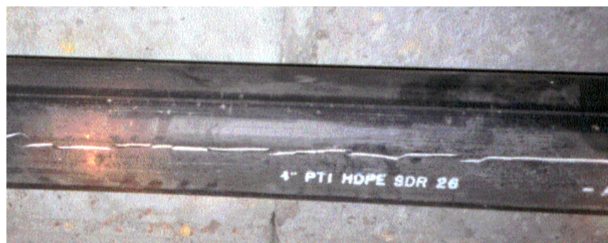
Figure 4. Typical cracking of the PE duct.
