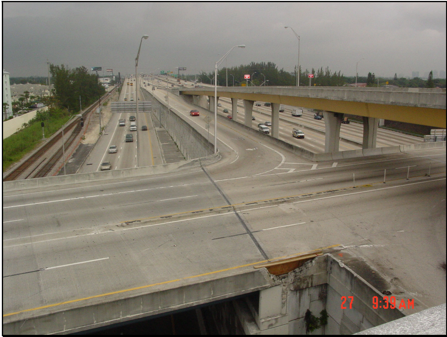
Figure 3. Looking north into the intersection of SB I-95 off-ramp at SR 84. Note damaged concrete wall on the south side.
