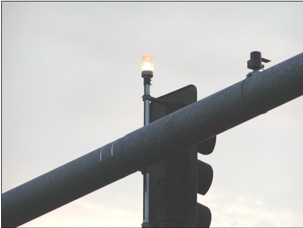
Photo 1: Typical Installation of a White Enforcement Light
