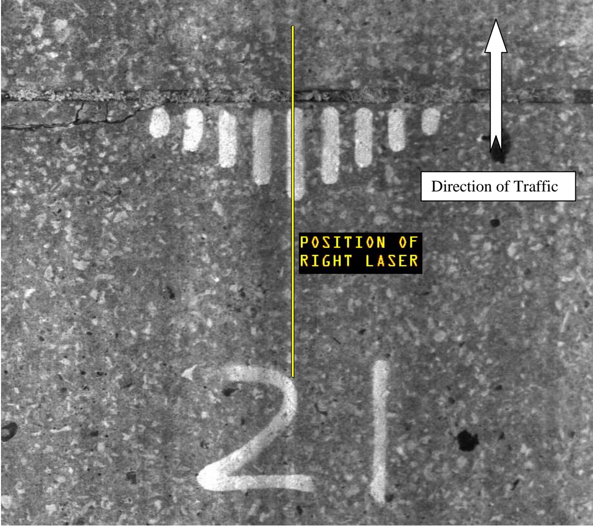
FIGURE 5 Matching of right laser lateral position with Faultmeter test location
