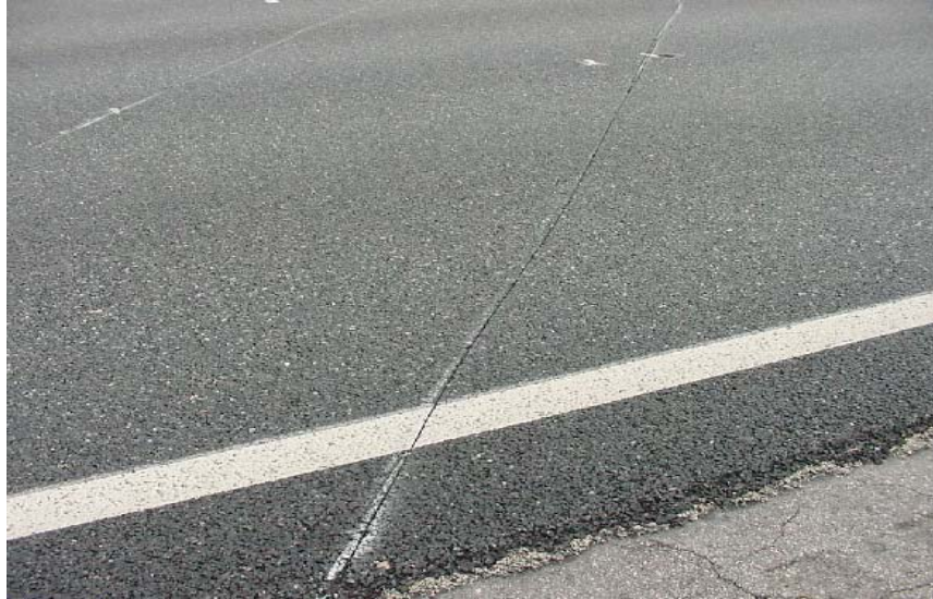
FIGURE 11 Transverse Angled Grooves as a Short-term Solution to Water Drainage Problem
