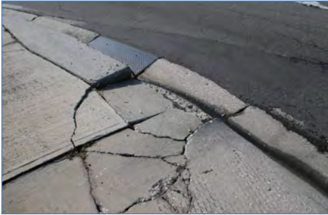
Damaged pavement is common in the Tampa Bay region due to inadequate truck turn radii at intersections.
