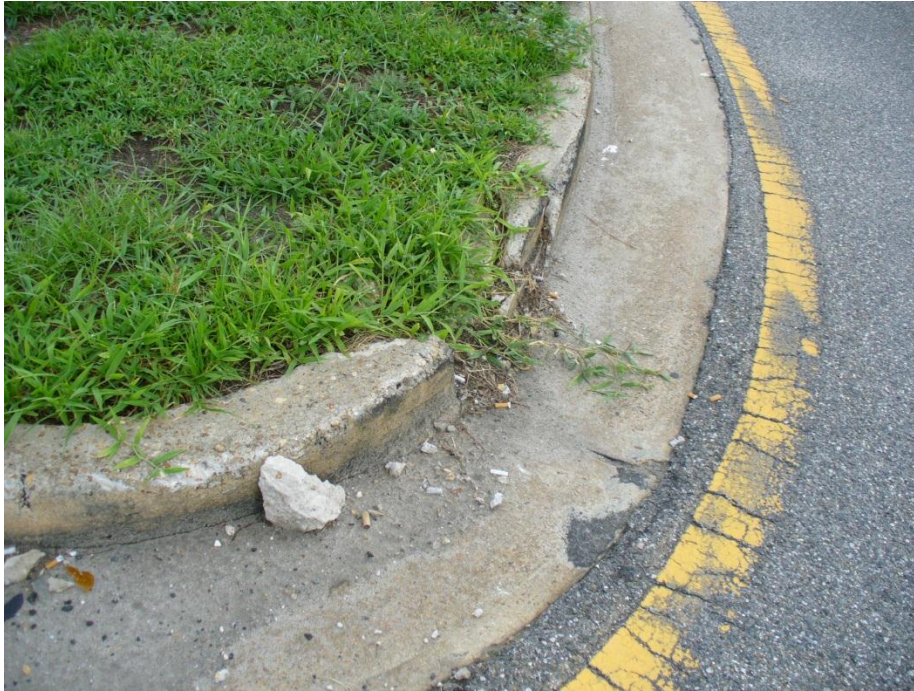
Photo 6 Curb damage caused by off-tracking trucks.
