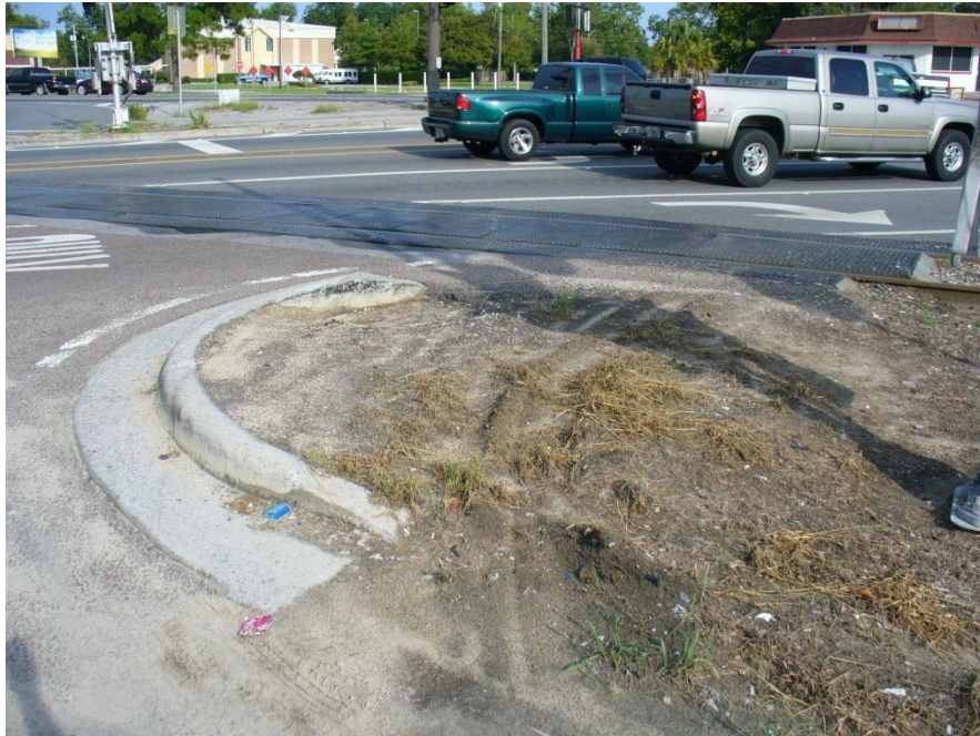
Photo 5 Shoulder rutting at Lafayette Road. Curb appears to serve no useful purpose.
