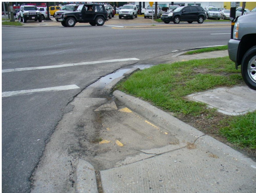
Photo 5 Curb damage caused by off-tracking trucks at the southeast corner of US 98 and Harrison Avenue.
