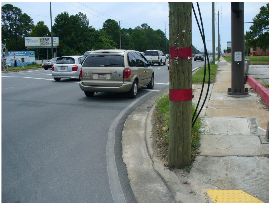
Photo 6 Pole at the northwest corner is too close to roadway.
