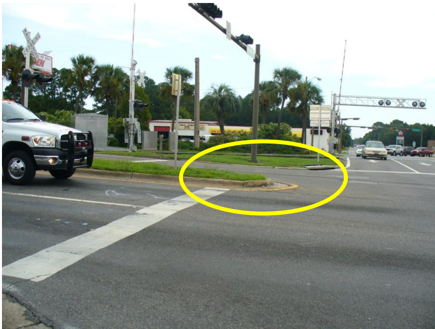
Photo 7 Bull nose damage on US 98 at Harrison Avenue
