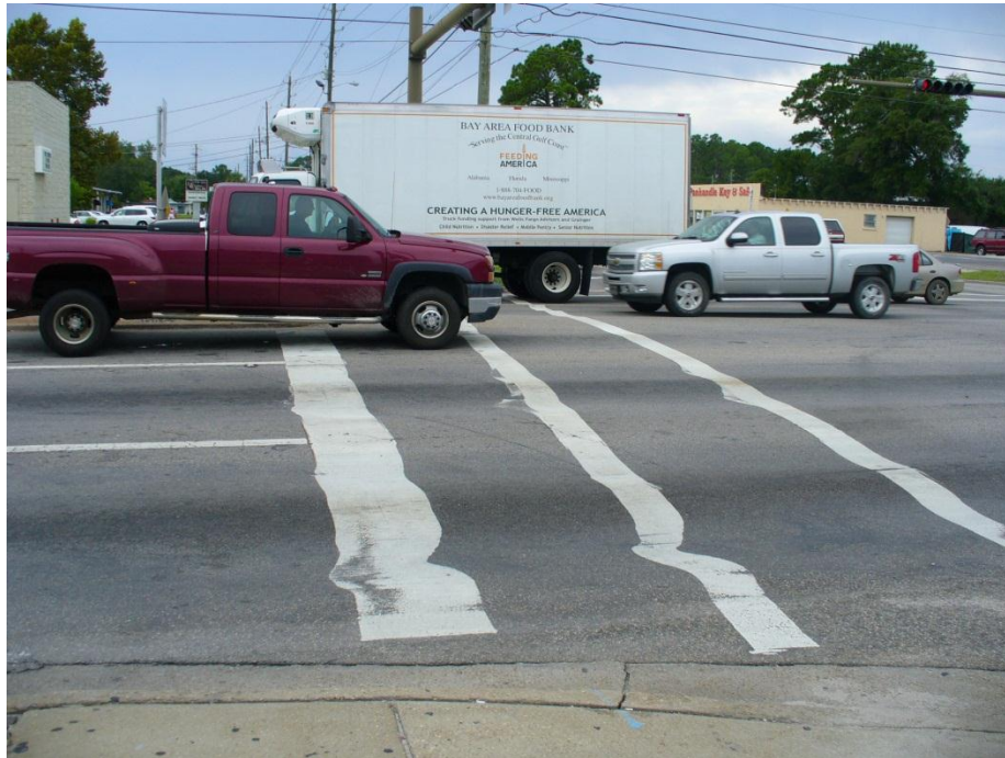
Photo 2 Deep rutting in westbound lanes of US 98 at Jenks Avenue
