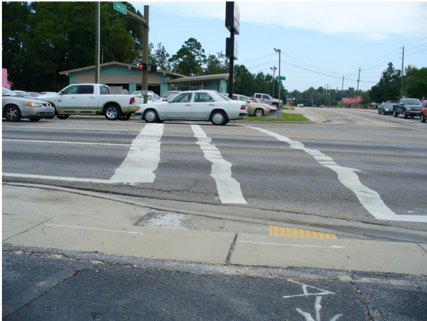
Photo 1 Deep rutting and some minor cracking in all eastbound lanes on US 98 at Jenks Avenue.
