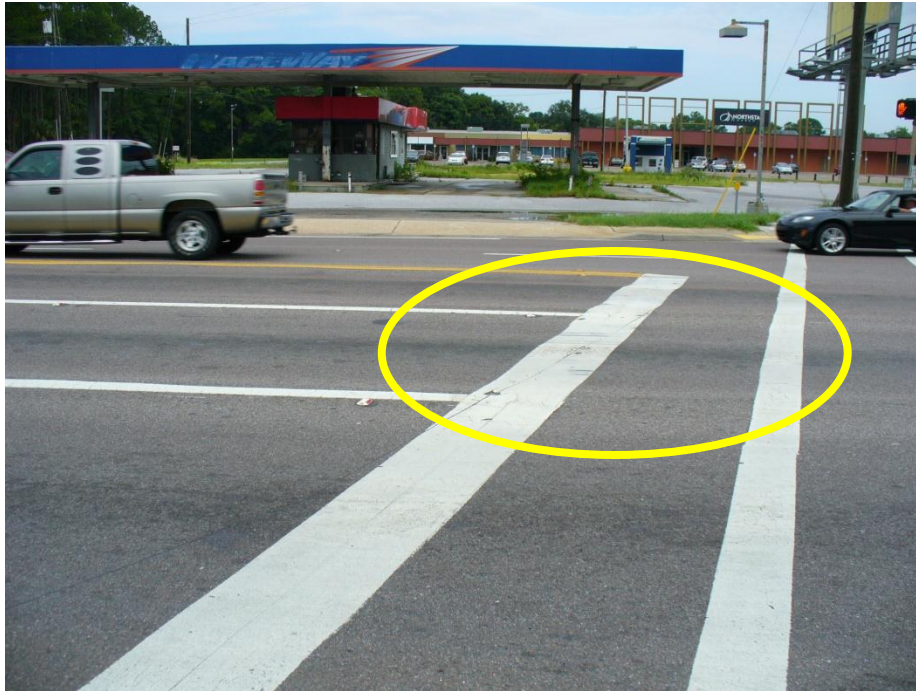
Photo 1 Minor rutting on the SR 368 (23 rd Street) eastbound approach
