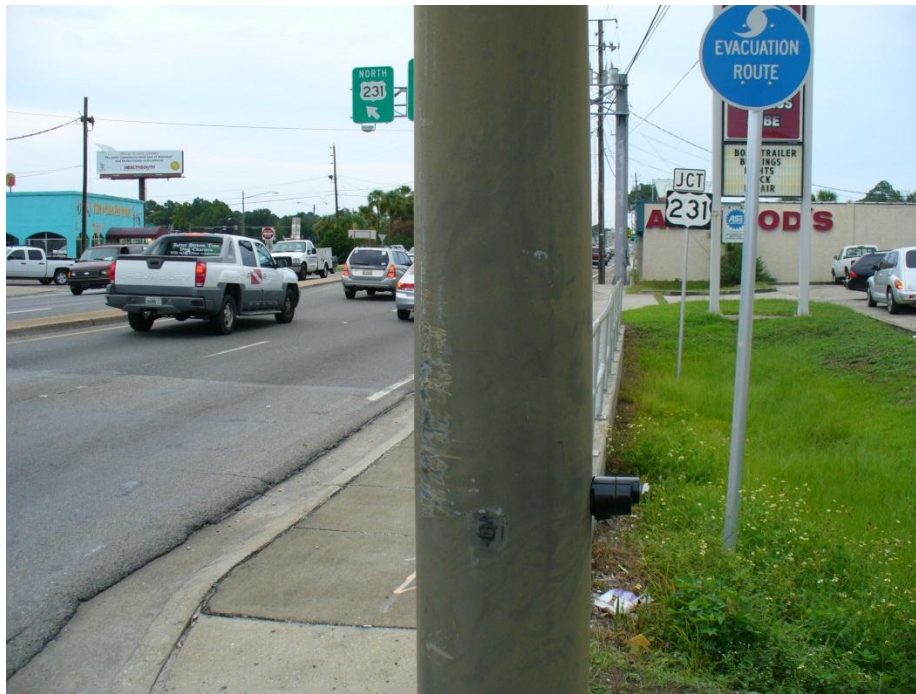
Photo 4 Mast arm damage caused by turning truck at the southeast corner of US 98/Jenks Avenue intersection.
