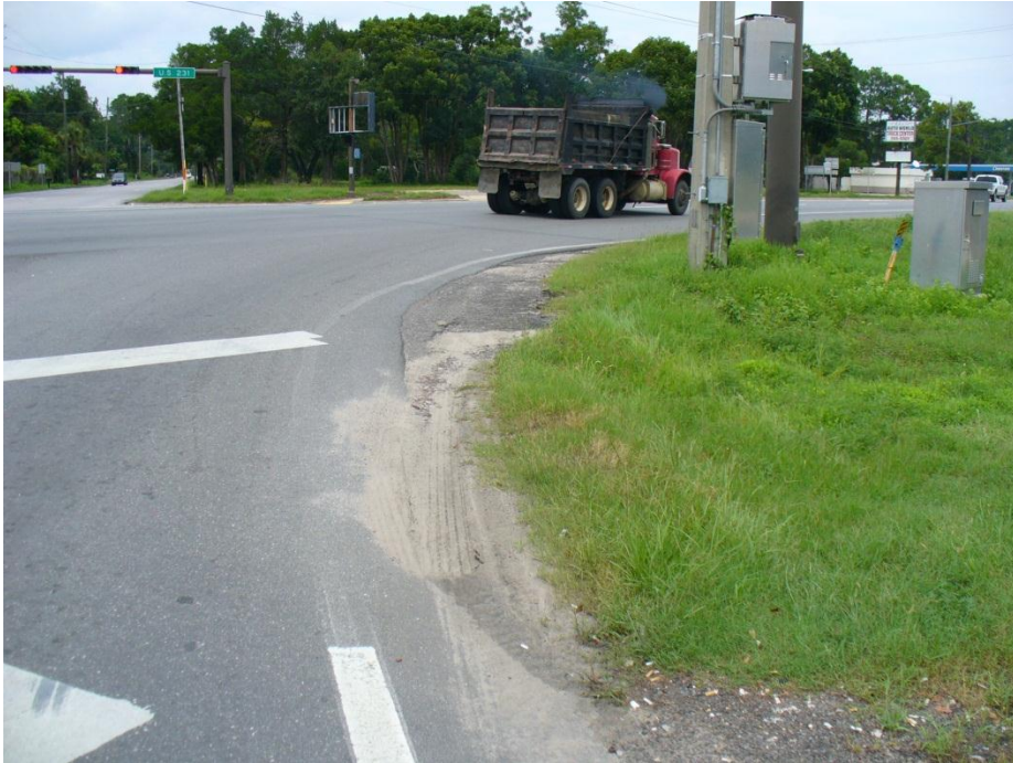
Photo 1 Northeast corner is heavily rutted and the shoulder pavement is deteriorating.
