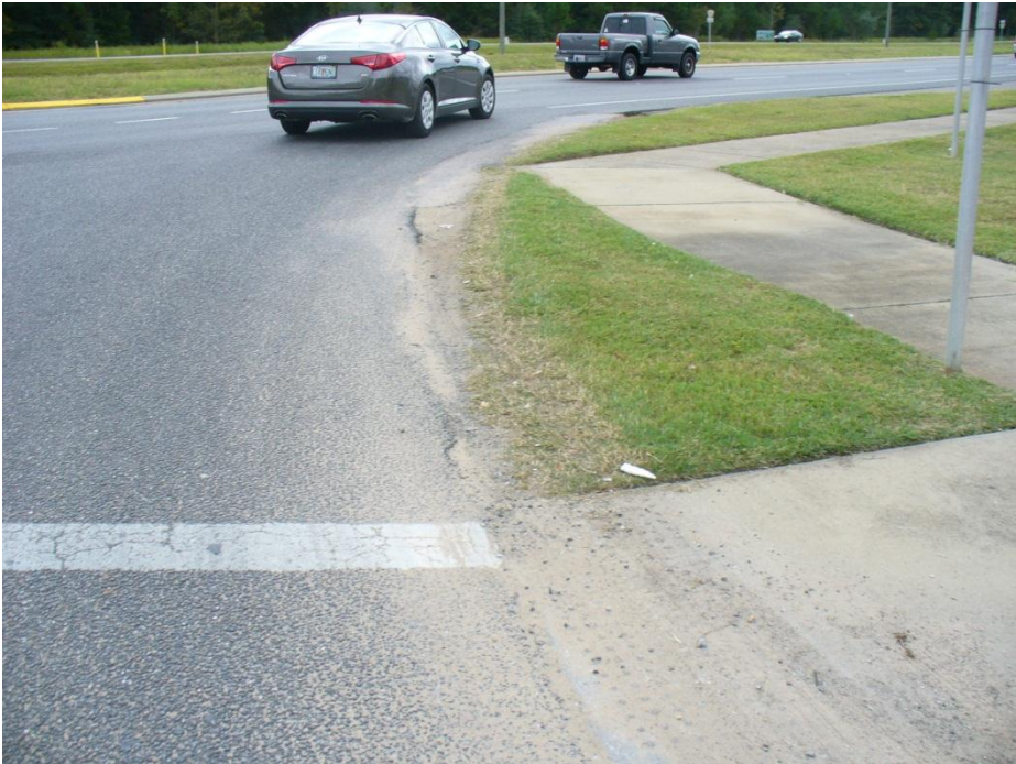
Photo 10 Sidewalk from southwest corner of Airport Road extending south on west side of SR 85
