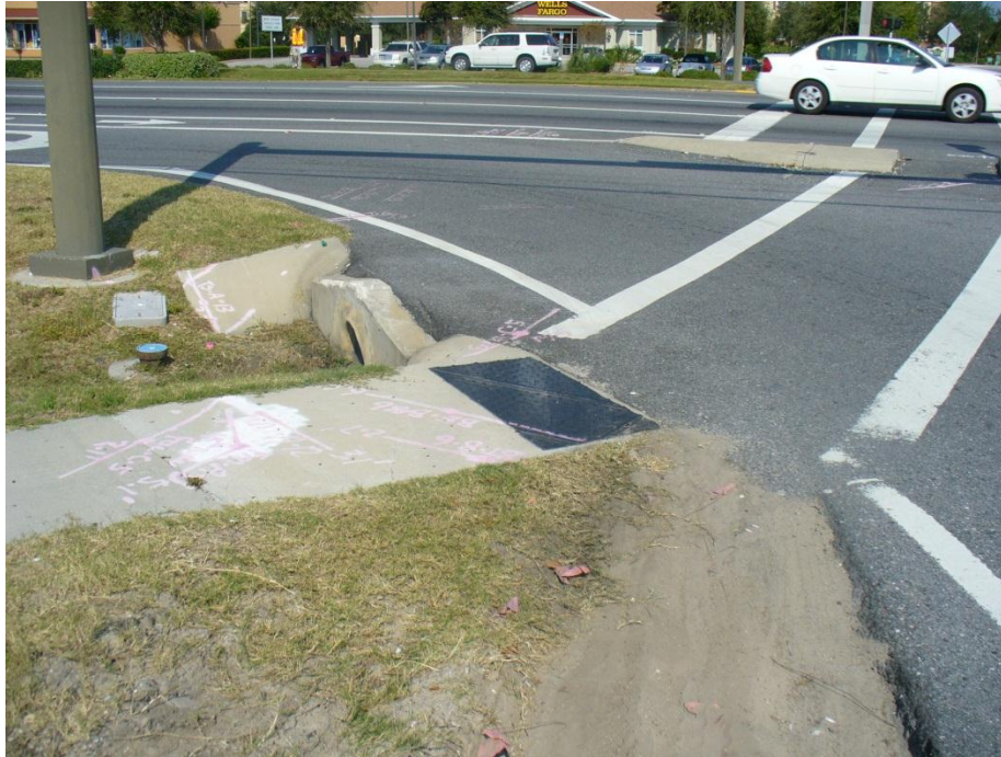
Photo 5 Southwest corner of Matthew Boulevard showing unsafe concrete culvert and sidewalk
