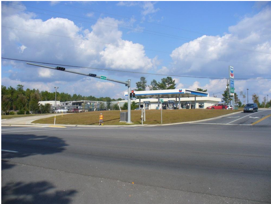
Photo 6 New signal at Business Park Road (looking northeast)
