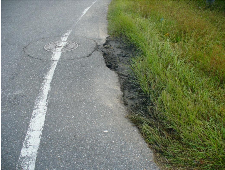
Photo 1 Soft shoulder damage at southeast corner of John King Road
