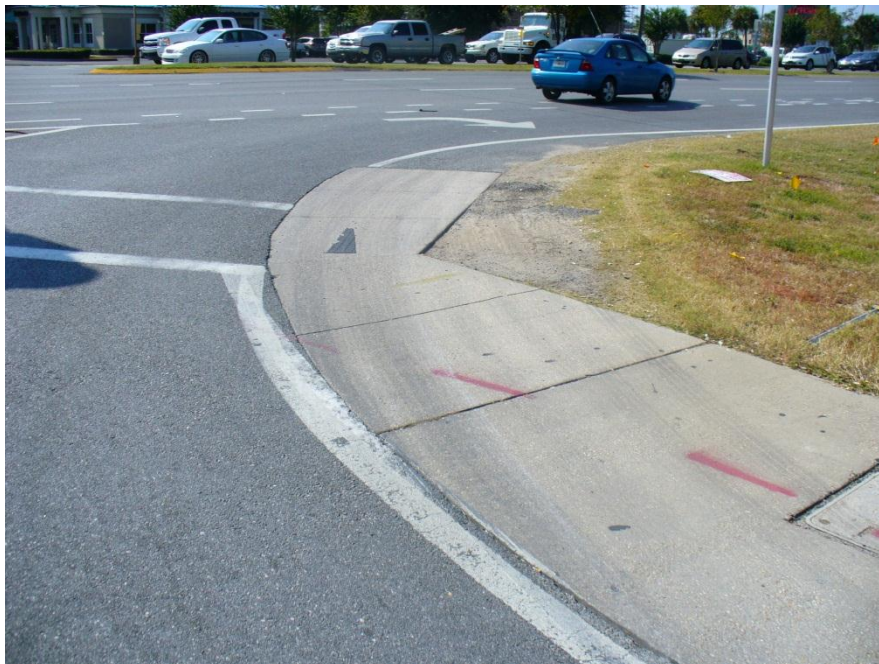
Photo 6 Danny Wuerffel Way showing off-tracking. The sidewalk is truck mountable but should be extended to include the rutted area.
