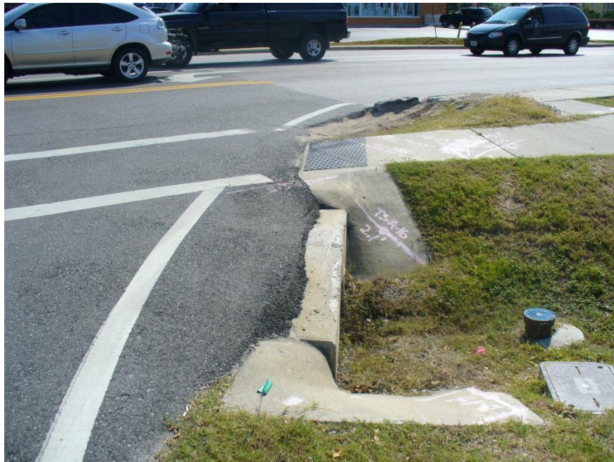
Photo 4 Matthew Boulevard safety issues. The culvert should be extended further away from the EOP or a guardrail installed to prevent trucks leaving the road and over-turning.
