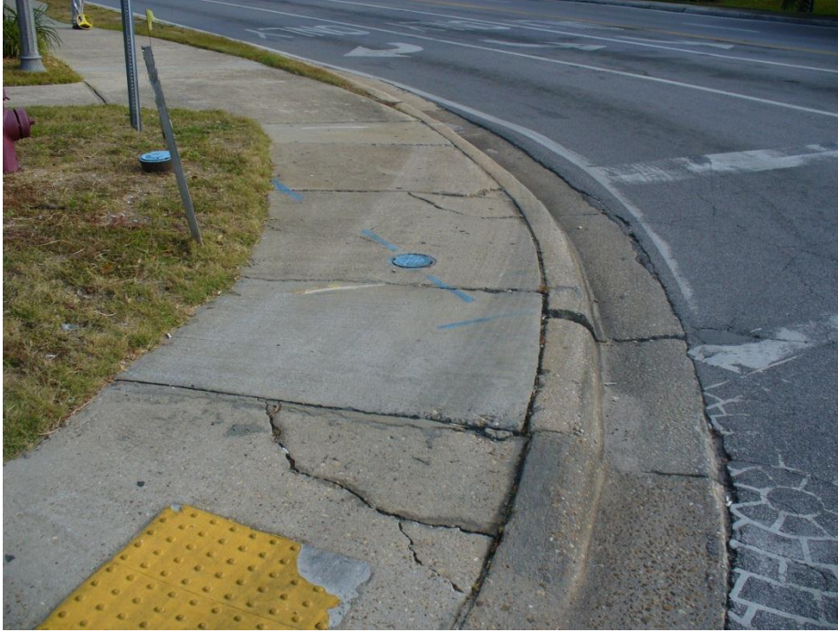
Photo 3 Cracked sidewalk caused by off-tracking trucks at Main Street
