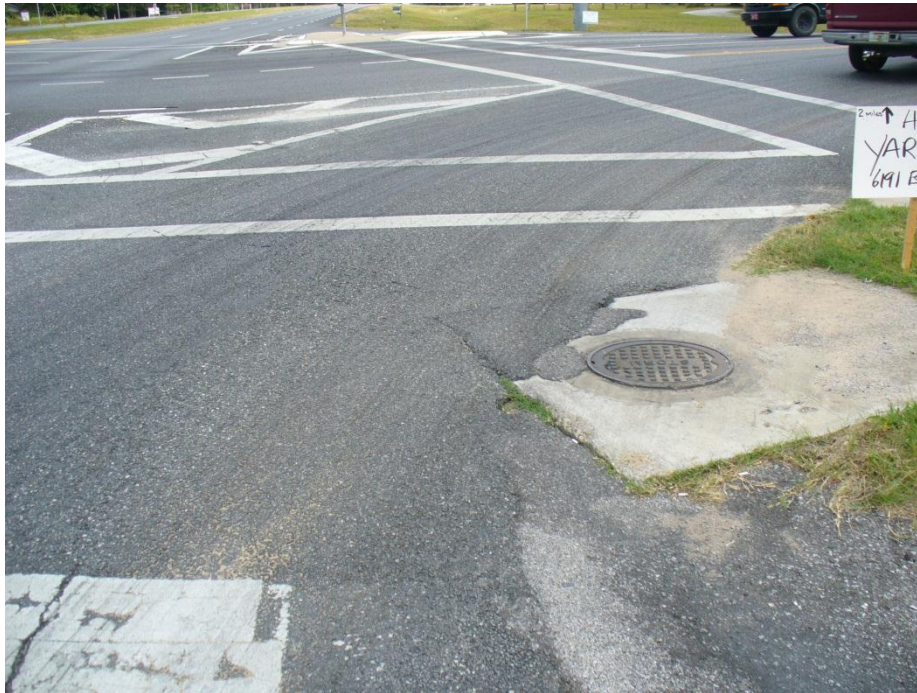
Photo 11 Damaged storm drain at the southeast corner of Airport Road
