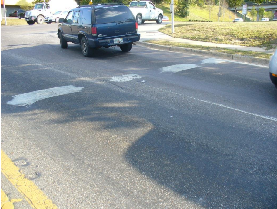
Photo 3 Deep rutting in the eastbound lanes of US 90 at US 331 South
