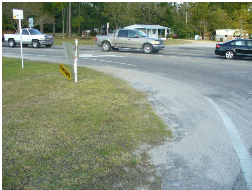
Photo 4 Shoulder deterioration due to off-tracking at the northwest corner of US 331 and US 90
