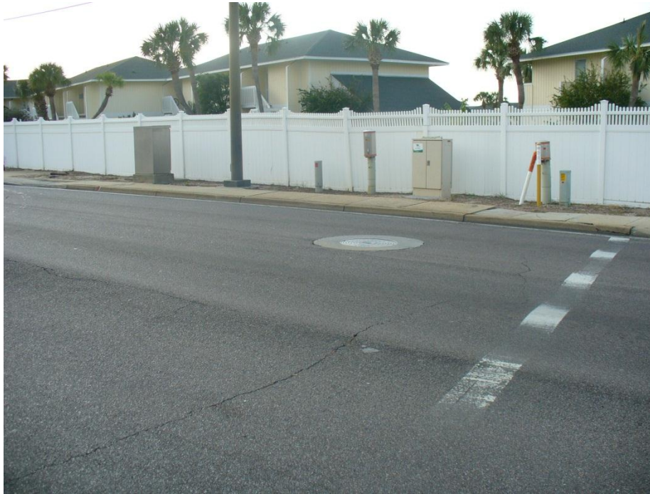
Photo 1 Through lane rutting was noted at intersections in Segments 1-3 of the corridor. This photo shows rutting at Main Street.
