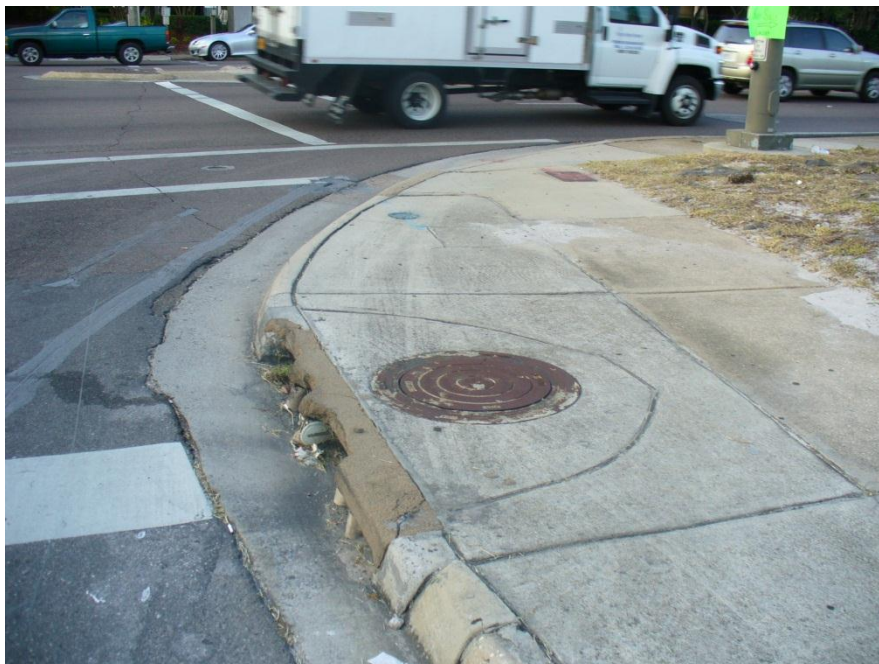
Photo 2 Off-tracking indicated by the damaged storm drain and tire tracks on the sidewalk at Beach Drive
