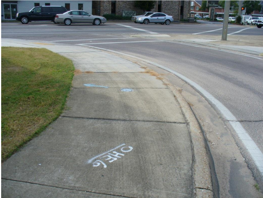
Photo 5 Tire marks from off-tracking trucks at northeast corner of US 90 and SR 85
