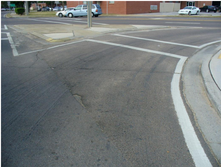
Photo 4 Channelized right-turn lane at northeast corner of US 90 and SR 85, note the raised concrete pedestrian island and cracked pavement
