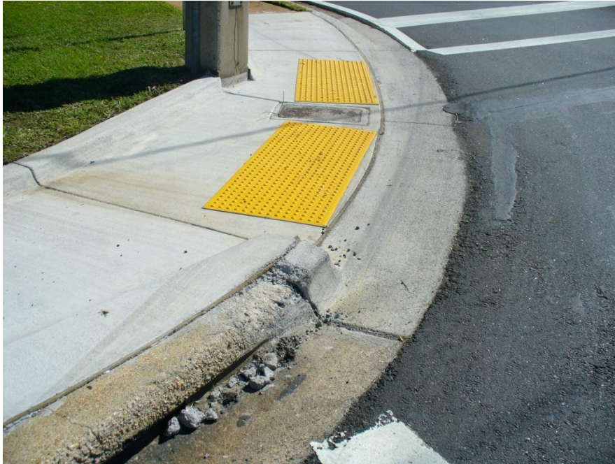
Photo 11 Damaged curb at W. Fairfield Drive due to over tracking
