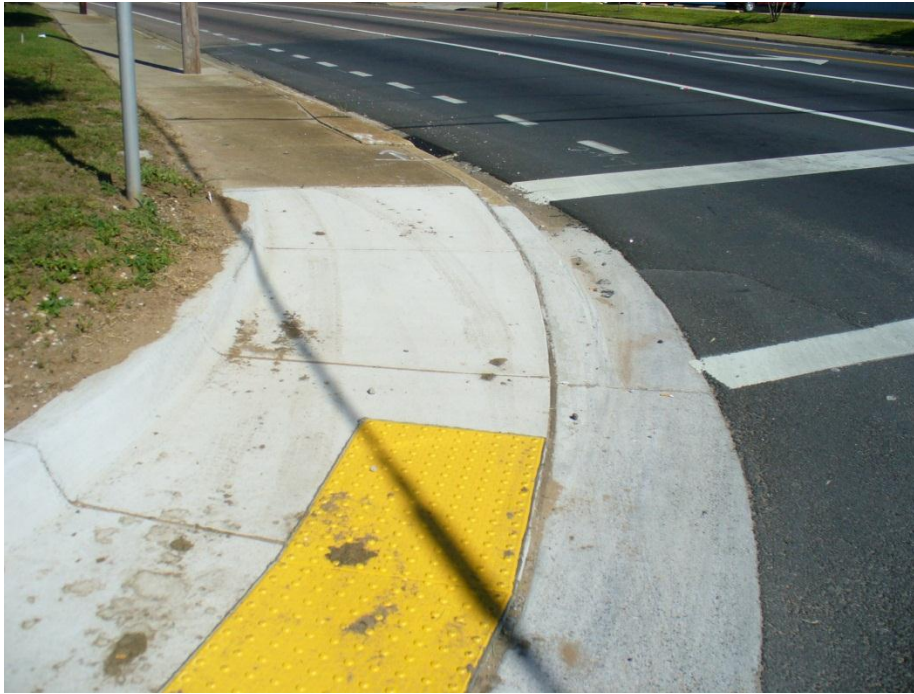
Photo 5 Tire tracks on recently modified pedestrian ramp on W. Fairfield Drive, similar conditions were noted at all quadrants
