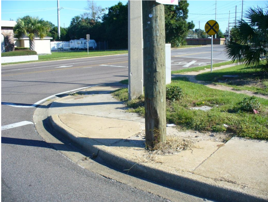
Photo 3 Damaged pole at the southeast corner of W. Leonard Street
