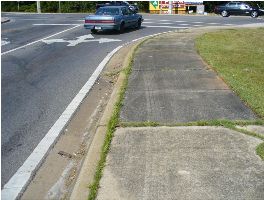
Photo 11 Northbound to eastbound right turn at Ward Basin Road showing tire marks from truck off-tracking
