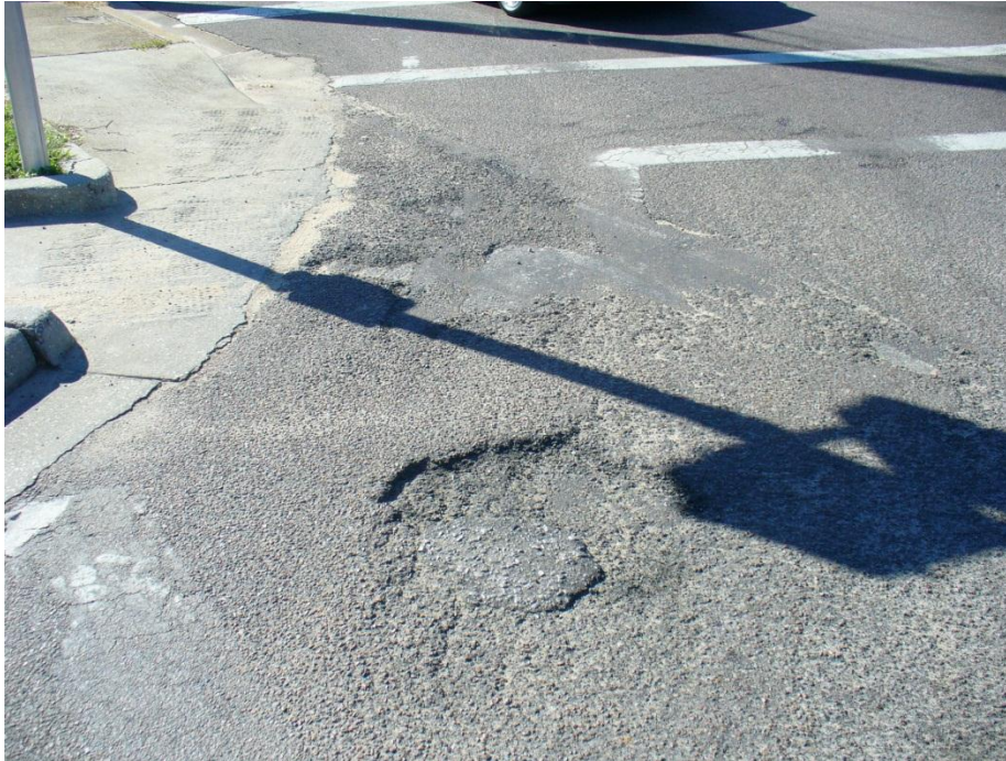
Photo 1 Rough pavement and pothole southeast quadrant at W. Texar Drive
