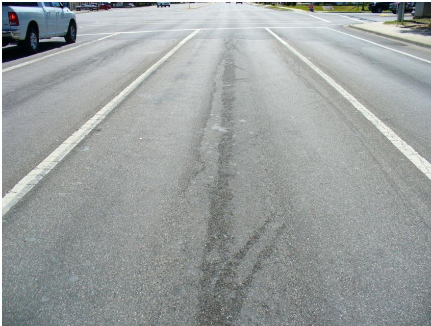
Photo 2 Rutting on southbound approaches to E. Brent Lane
