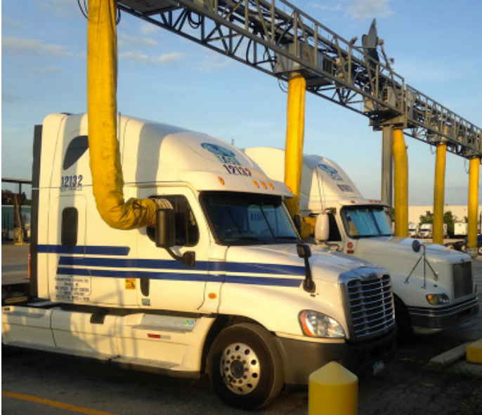
Single-System Truck Parking Electrification System
