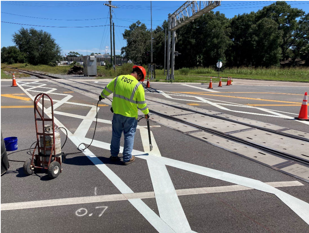
A dynamic envelope being installed at DOT #713448R, South Byron Butler Parkway
