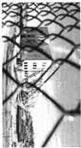
A new school is under construction in Boca Raton on Dec. 7. Some parents at Thursday's Advisory Board meeting Committee meeting called for more studies so families can weigh a variety of options and configurations for redefining boundaries. CAROL KATZ/SOUTH FLORIDA SUN SENTINEL
