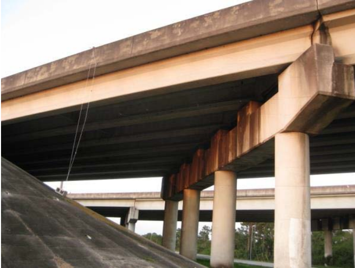
Bridge stained with bat guano
