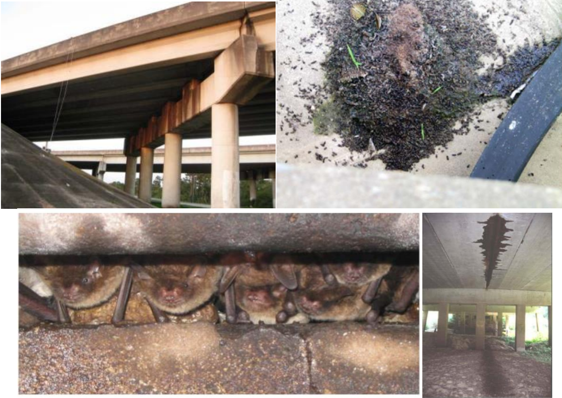
Top Left – Bridge staining. Top Right – Guano deposits visible from bridge deck. Bottom Left – Visible bats within an expansion joint. Bottom Right – Staining on underside of expansion joint and guano deposits on the ground.
