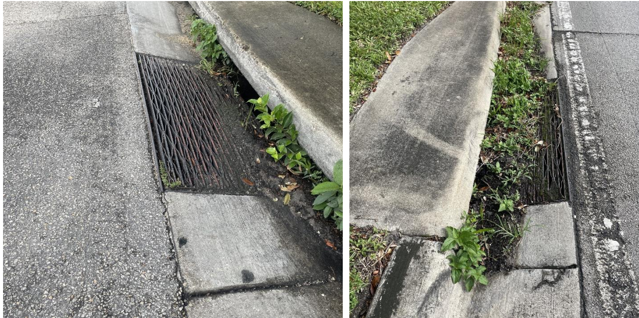
Figure 2-6 Existing Drainage Issues
