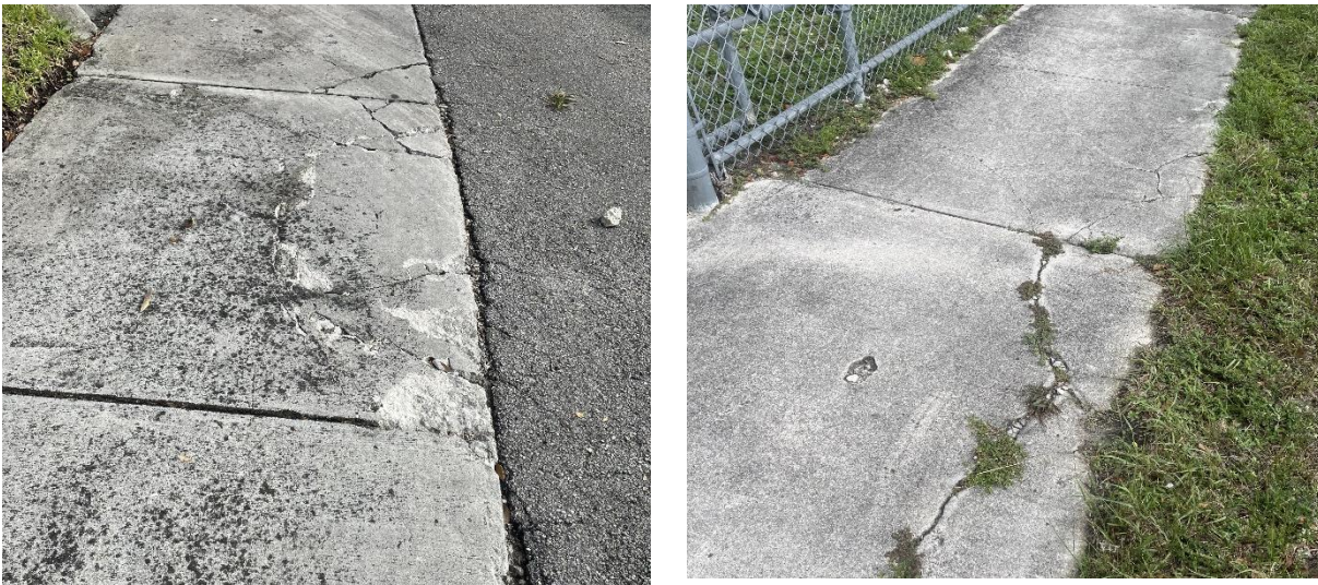
Figure 2-7 Damaged or Uneven Sidewalks
