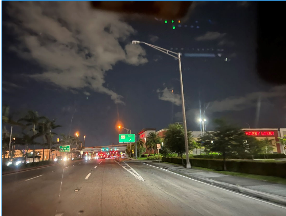
Photo 12 – Non-functioning luminaire east of W 20 th Ave (north side of SR 932/NW 103 rd Street)
