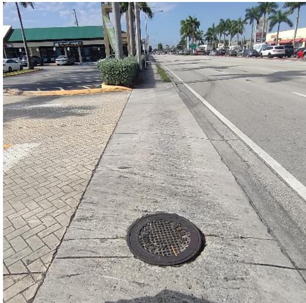
Photo 19: Looking at the driveway east of the southeast corner of West 8 Avenue.
