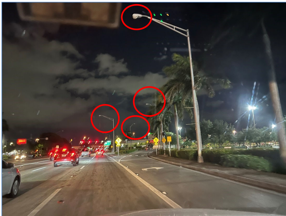
Photo 11 – Non-functioning luminaires east of W 18 th Ct (north side of SR 932/NW 103 rd Street)
