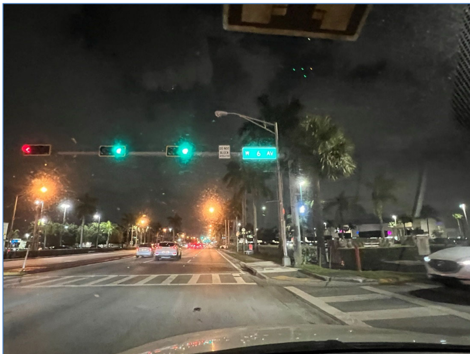
Photo 7 – Non-functioning luminaire east of W 6 th Ave (south side of SR 932/NW 103 rd Street)
