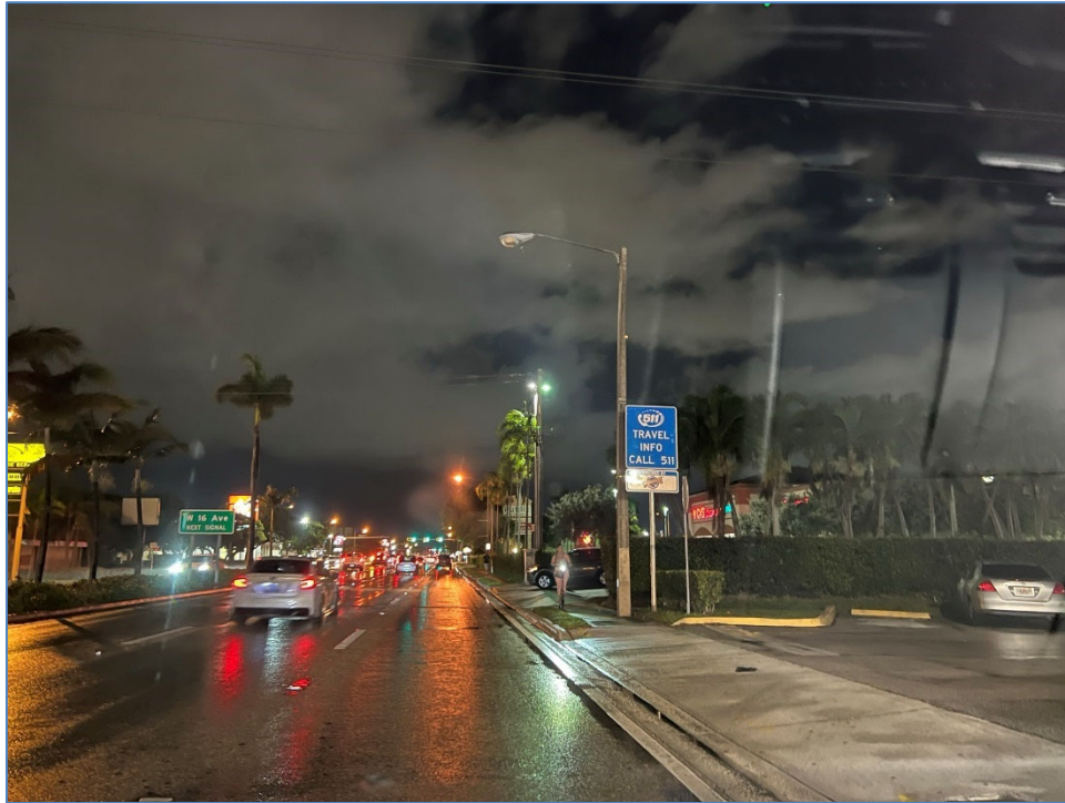
Photo 10 – Non-functioning luminaire east of W 16 th Ave (north side of SR 932/NW 103 rd Street)
