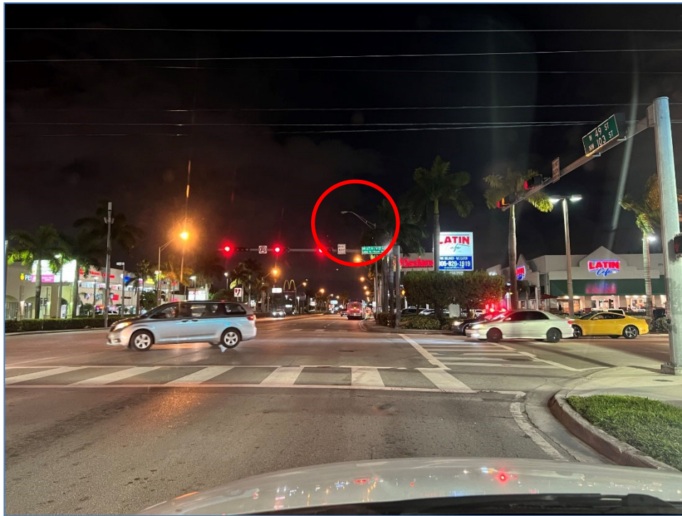
Photo 4 – Non-functioning luminaire east of Ludlam Rd (south side of SR 932/NW 103 rd Street)
