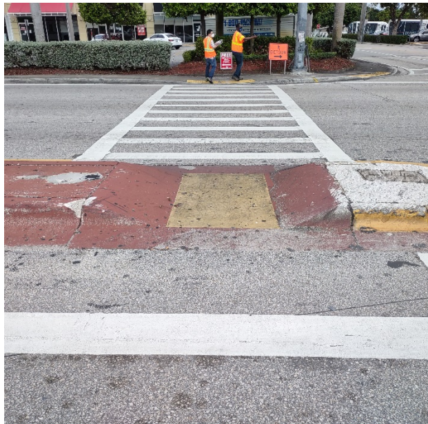
Photo 51: Traffic separator on the west leg crosswalk of West 10 Avenue.
