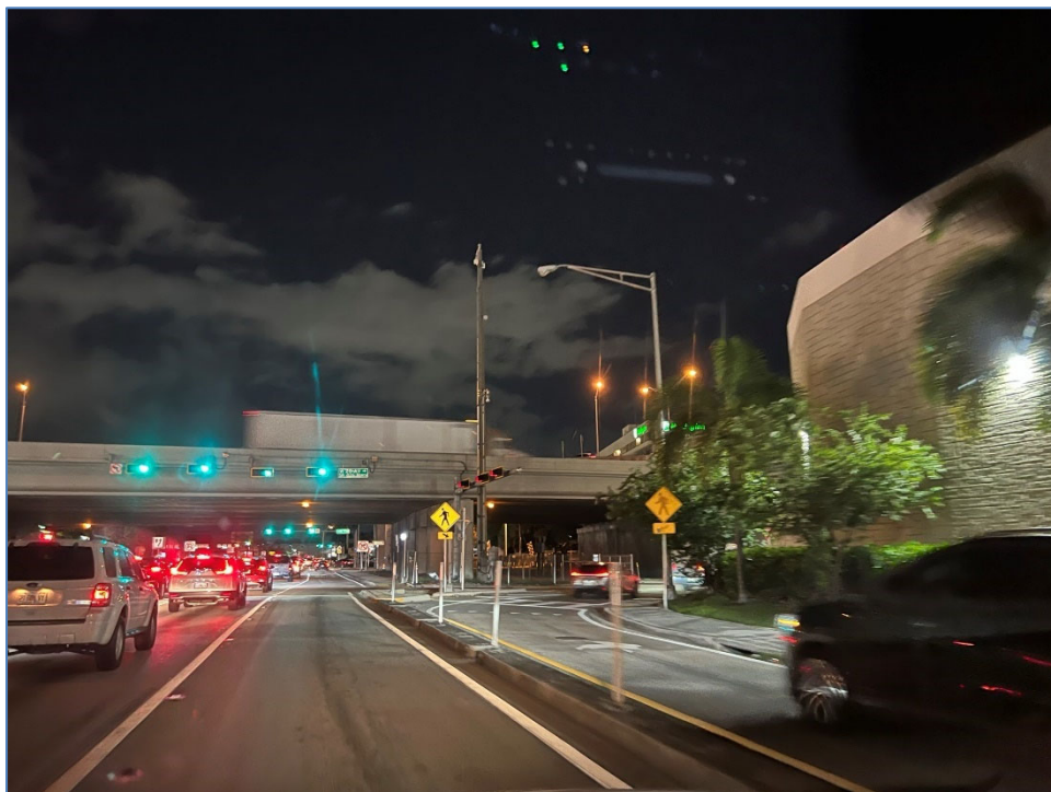
Photo 13 – Non-functioning luminaire east of W 20 th Ave (north side of SR 932/NW 103 rd Street)
