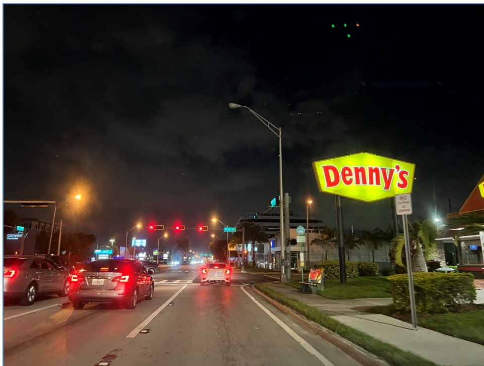
Photo 5 – Non-functioning luminaire west of W 10 th Ave (south side of SR 932/NW 103 rd Street)
