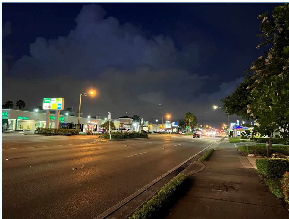
Photo 1 – Existing Street Lighting System (mostly HPS and sporadic LED)
