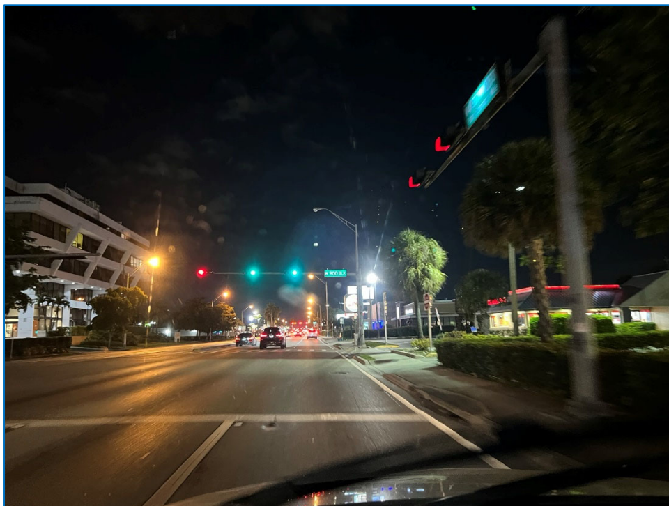
Photo 9 – Non-functioning luminaire west of W 900 Block (north side of SR 932/NW 103 rd Street)
