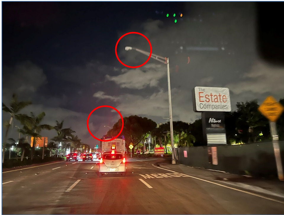
Photo 2 – Non-functioning luminaires east of W 20 th Ave (south side of SR 932/NW 103 rd Street); this includes luminaire not pictured to the west
