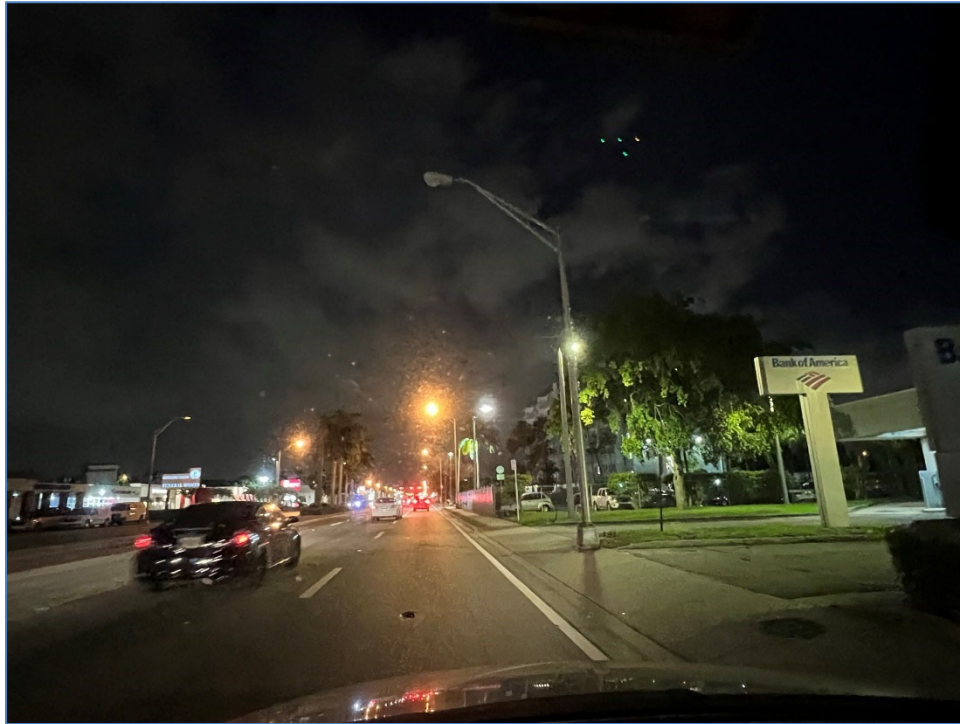
Photo 6 – Non-functioning luminaire east of W 900 Block (south side of SR 932/NW 103 rd Street)
