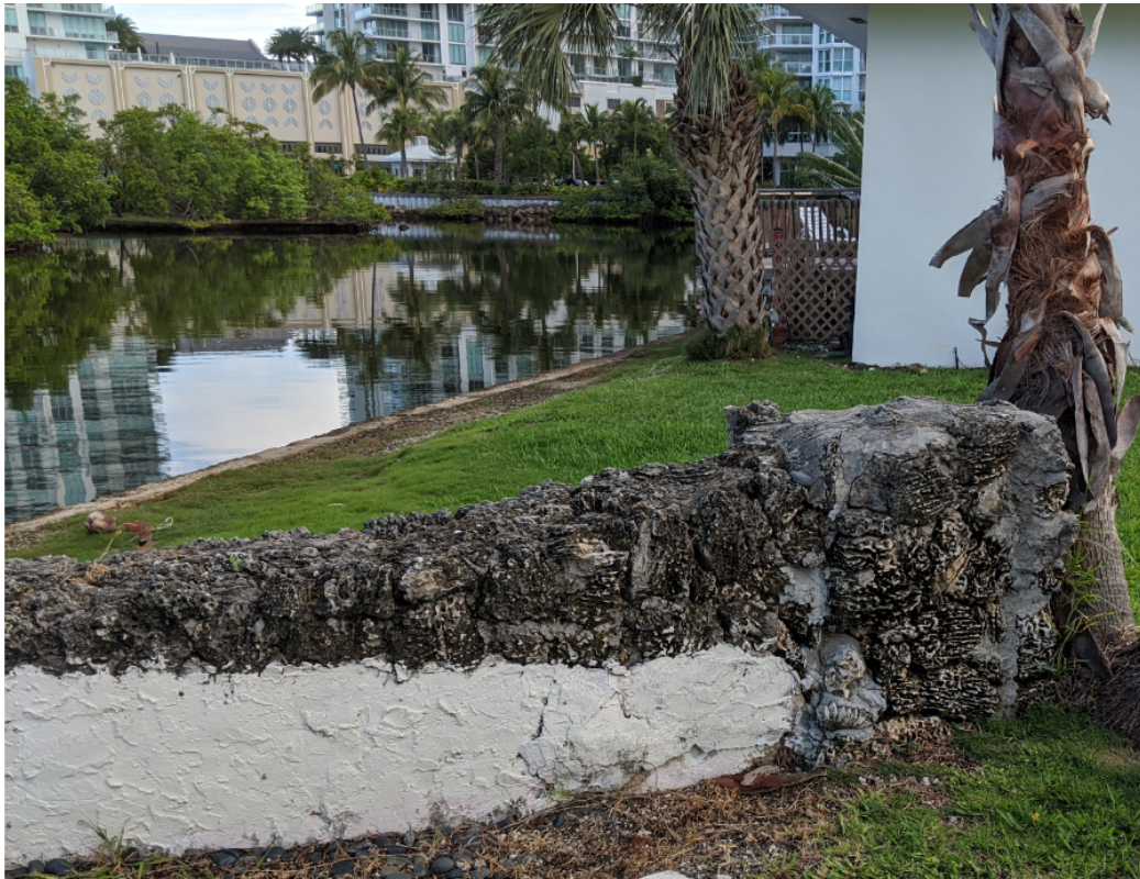
Figure 16: Coquina Limestone Rubble Attached to End of Parapet – NE Corner (1 of 2)
