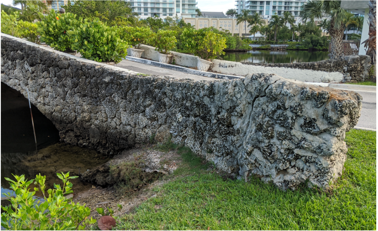
Figure 19: Cracked Coquina Limestone Rubble Attached to End of Parapet – SE Corner (2 of 2)
