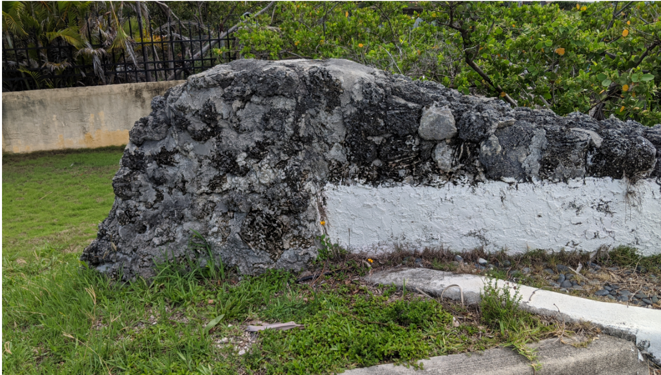
Figure 20: Coquina Limestone Rubble Attached to End of Parapet – NW Corner
