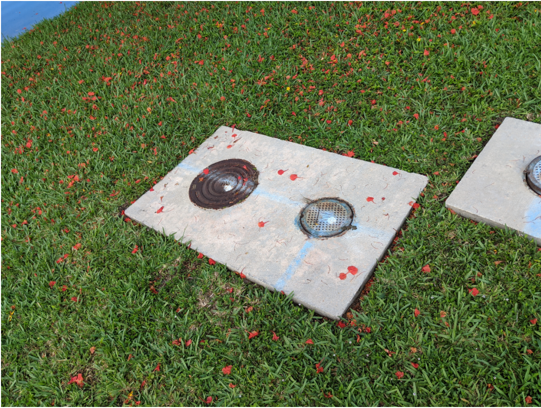
Figure 11: Water Valves – SW Corner (2 of 2)
