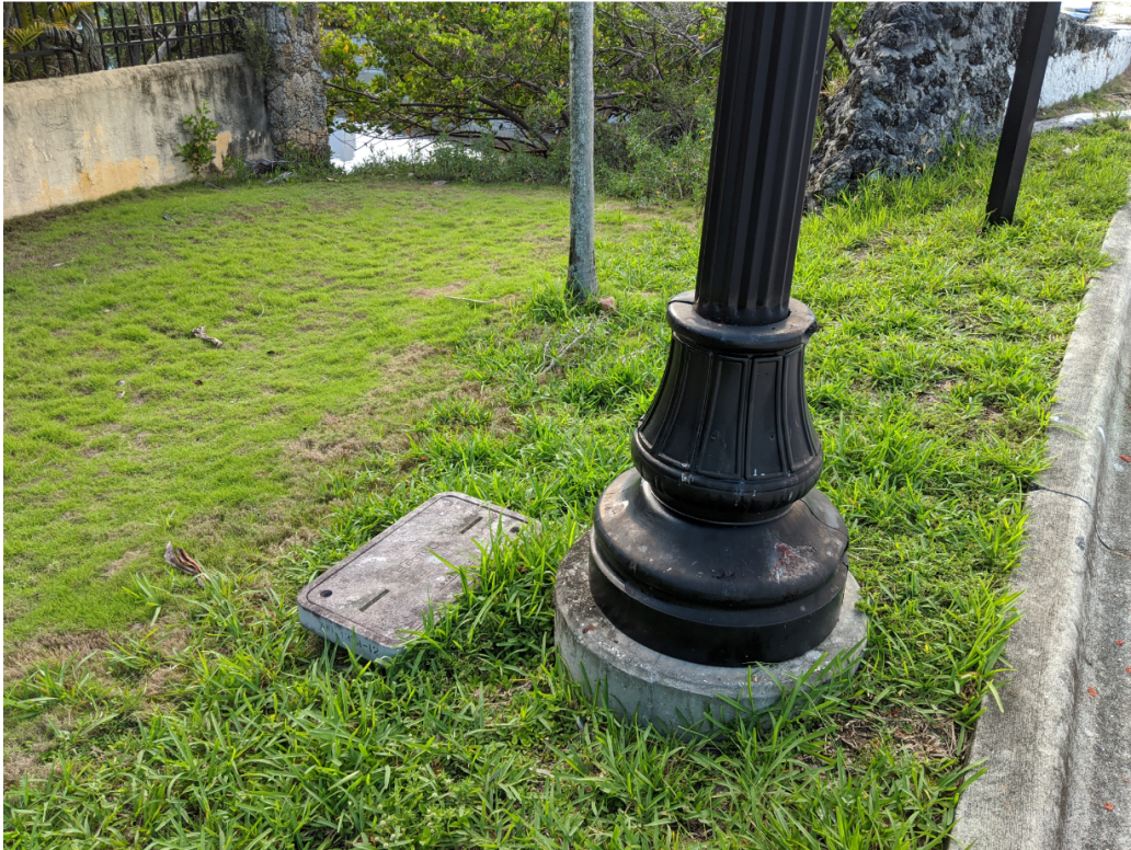
Figure 12: Electrical Pull Box with Light Pole and its Foundation – NW Corner.
