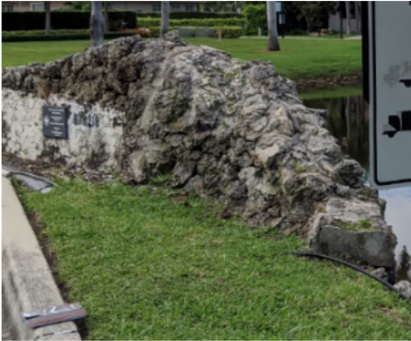
Figure 21: Coquina Limestone Rubble Attached to End of Parapet – SW Corner (1 of 2)
