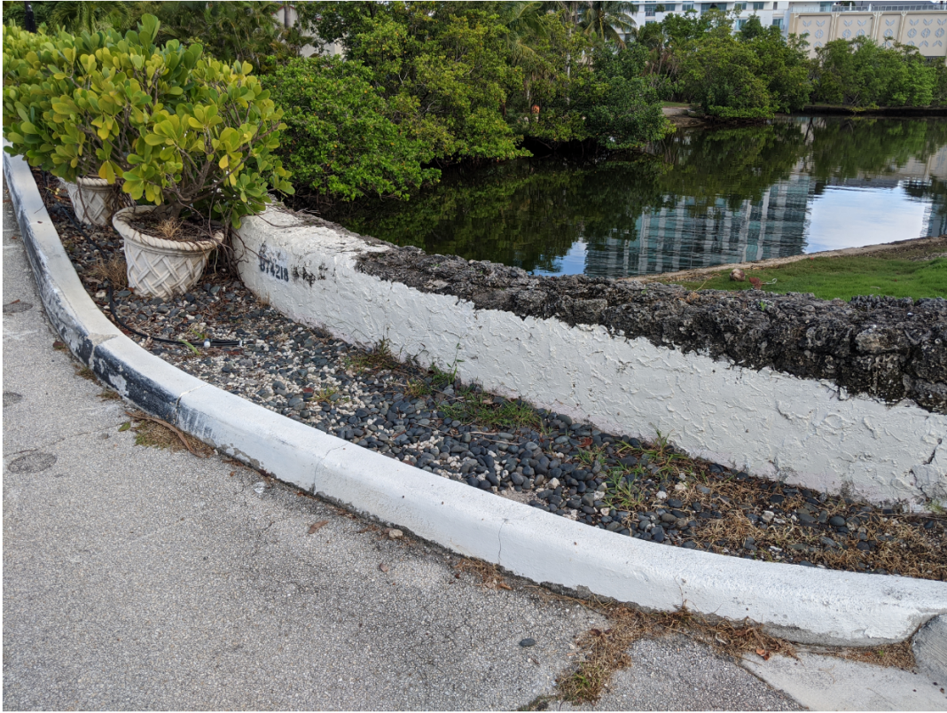
Figure 17: Coquina Limestone Rubble Attached to End of Parapet – NE Corner (2 of 2)
