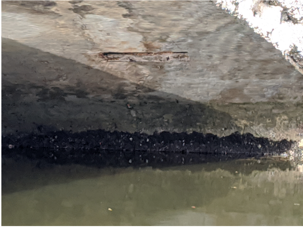
Figure 23: Damaged Stucco at Underside of Bridge Covered with Wooden Plank – Looking East
