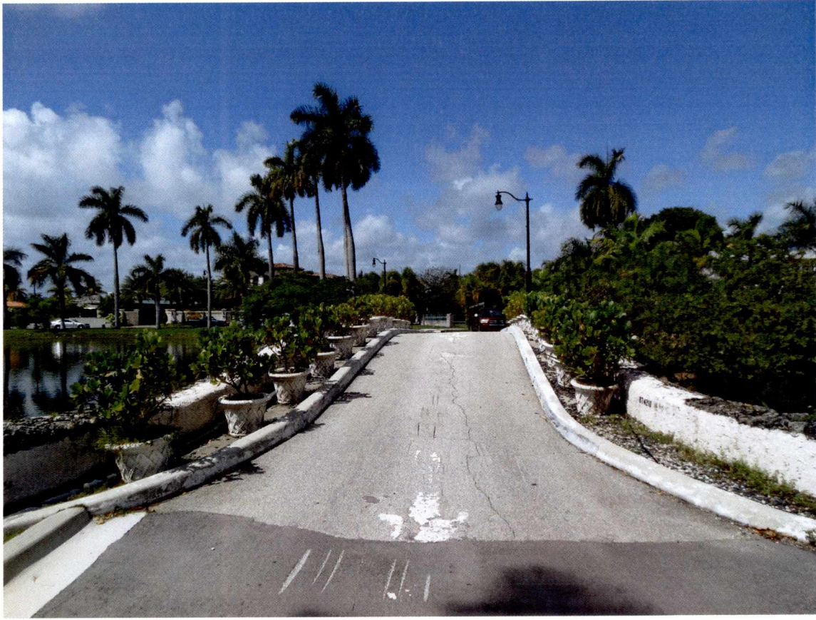
Longitudinal crack through asphalt on Bridge
