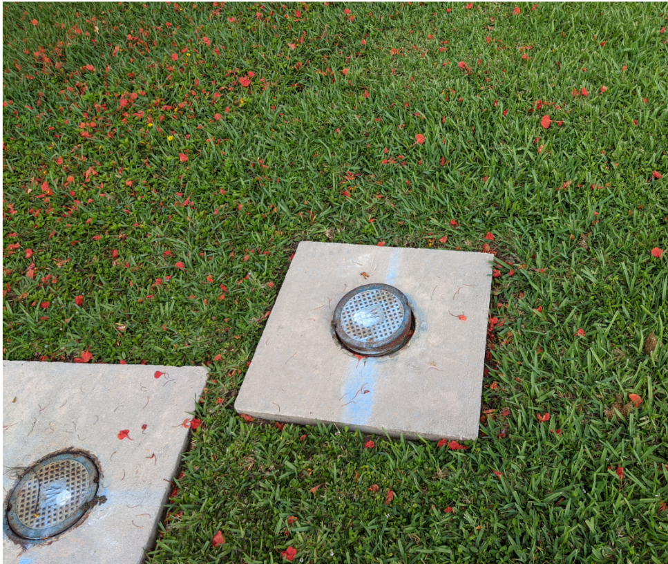
Figure 10: Water Valves – SW Corner (1 of 2)
