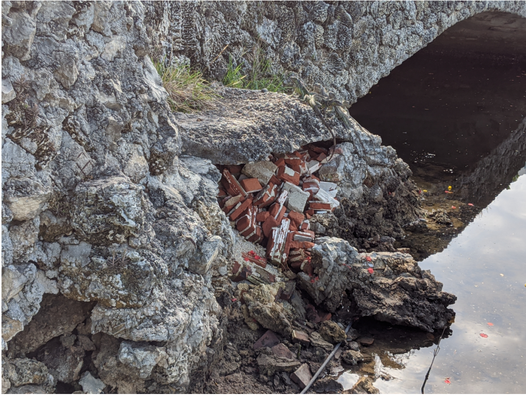
Figure 15: Damage to Western Abutment – Looking NE
