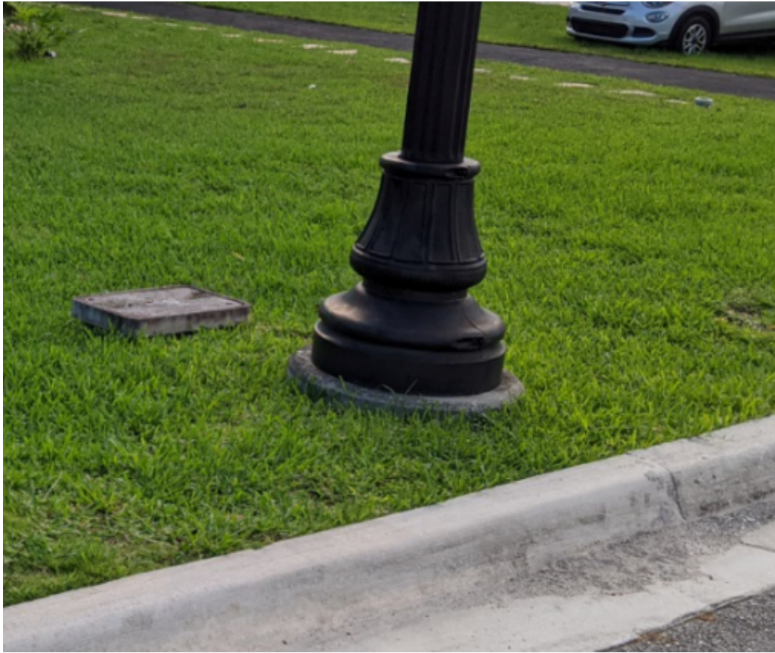
Figure 13: Electrical Pull Box with Light Pole and its Foundation – NE Corner.
