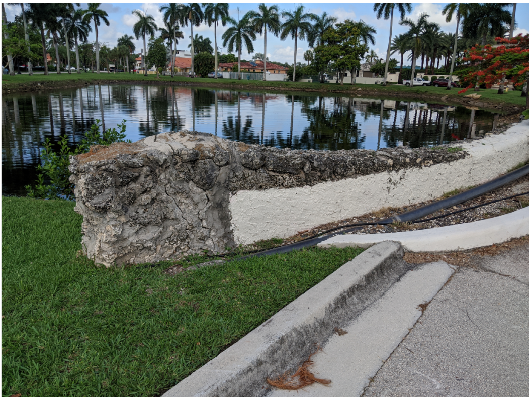
Figure 18: Cracked Coquina Limestone Rubble Attached to End of Parapet – SE Corner (1 of 2)
