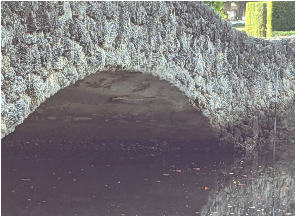
Figure 24: Damaged Stucco at Underside of Bridge Covered with Wooden Plank – Looking West
