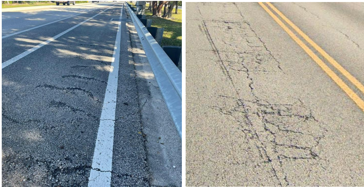
Figure 2-5 Existing Pavement Conditions
