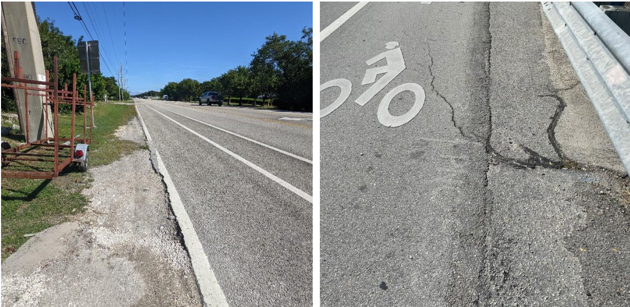
Figure 2-8 Damaged or Uneven Bike Path
