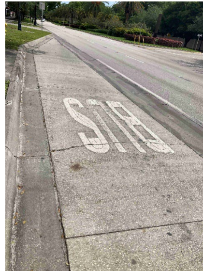
4. CRACKS ON PCC
