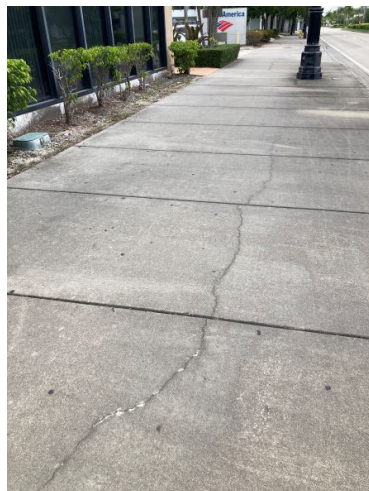
Cracks on sidewalk. Sta 143+00 LT
