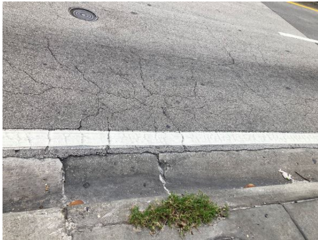
1. CRACKS ON ASPHALT
