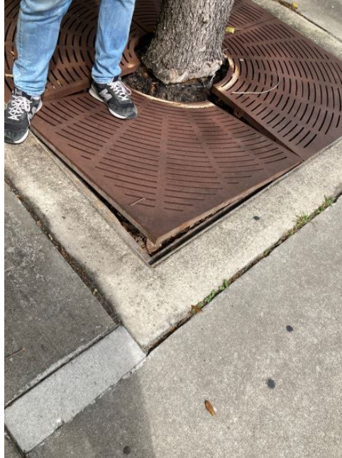
Tripping hazard. Typ.
