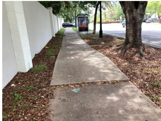
Uneven sidewalk. Sta 125+39 RT
