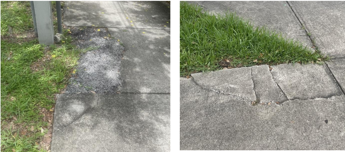
Figure 2-7 Damaged or Uneven Sidewalks
