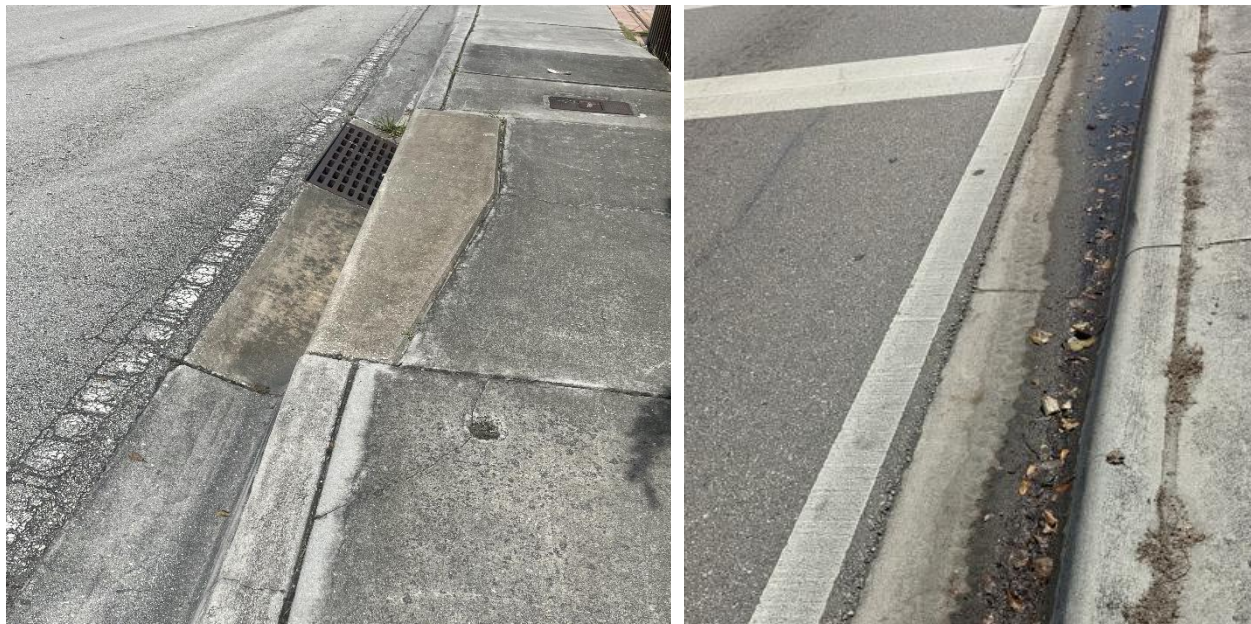
Figure 2-6 Existing Drainage Issues
