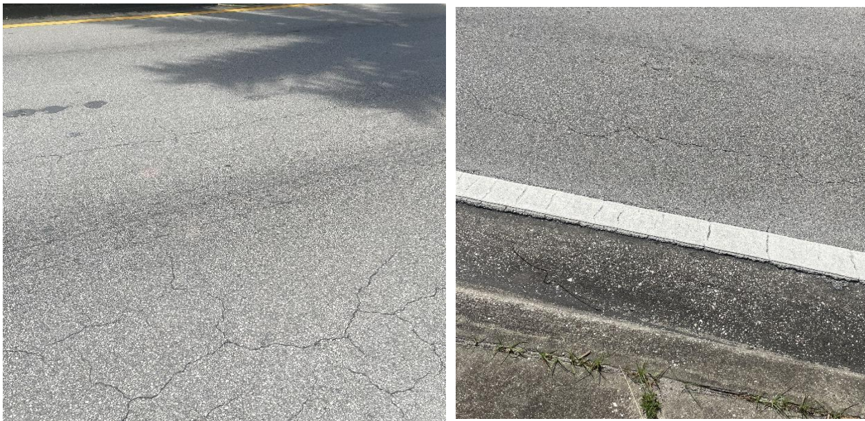
Figure 2-4 Existing Pavement Conditions
