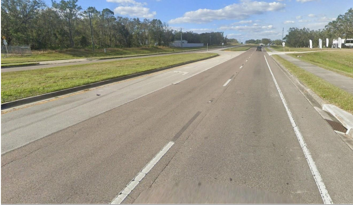
Figure 1: Existing turn lane 3,025 feet north of SR 64 in the northbound lanes of SR 35.
