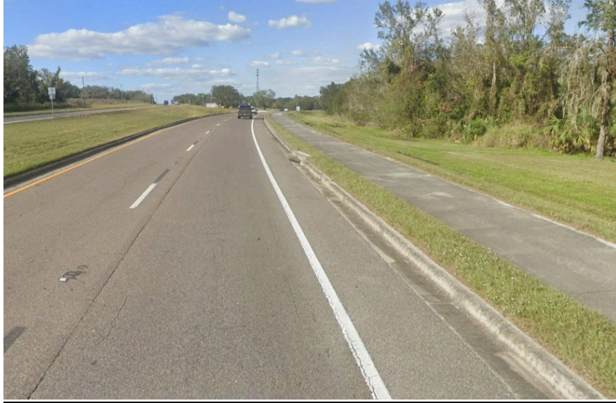
Figure 1: Existing median and outside Type F curb and 0-ft offset from the EOTW to median gutter lip and 4-ft offset from the EOTW to outside gutter lip on northbound SR 35.
