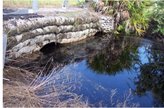
Sidedrain at cow pens, just north of bridge on S.R. 29. Ditch almost at capacity.
