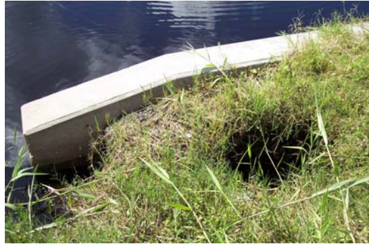
Erosion at headwall on east side of cross drain.
