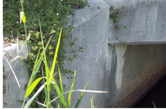
Water stains on west side of bridge.
