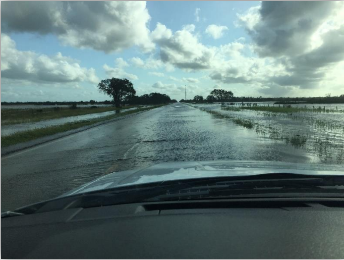
Figure 10: Hurricane Irma (2017) SR 29 Flooding Photo 1
