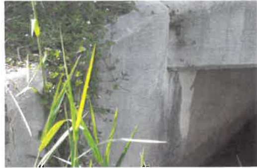
Water stains on west side of bridge.
