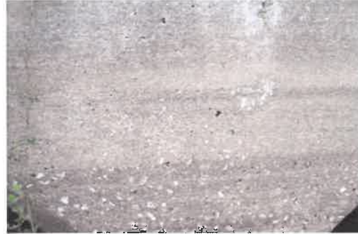
Water stains on headwall on west side of cross drain.
