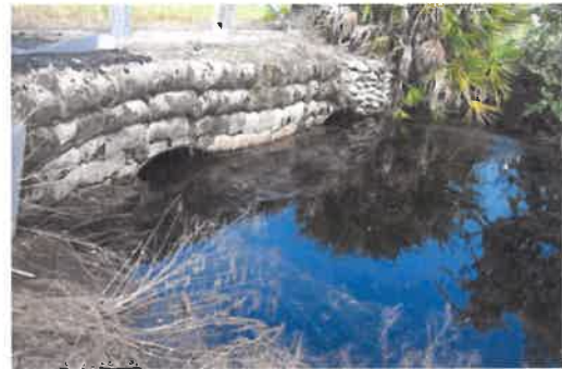
Sidedrain at cow pens, just north of bridge on S.R. 29. Ditch almost at capacity.
