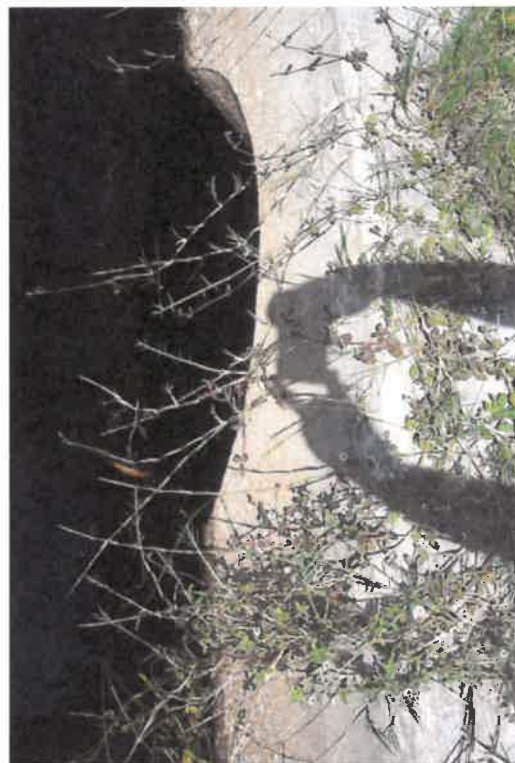
Staining on headwall on east side of cross drain.
