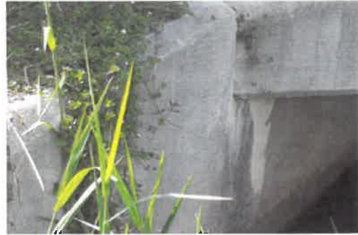
Water stains on west side of bridge.
