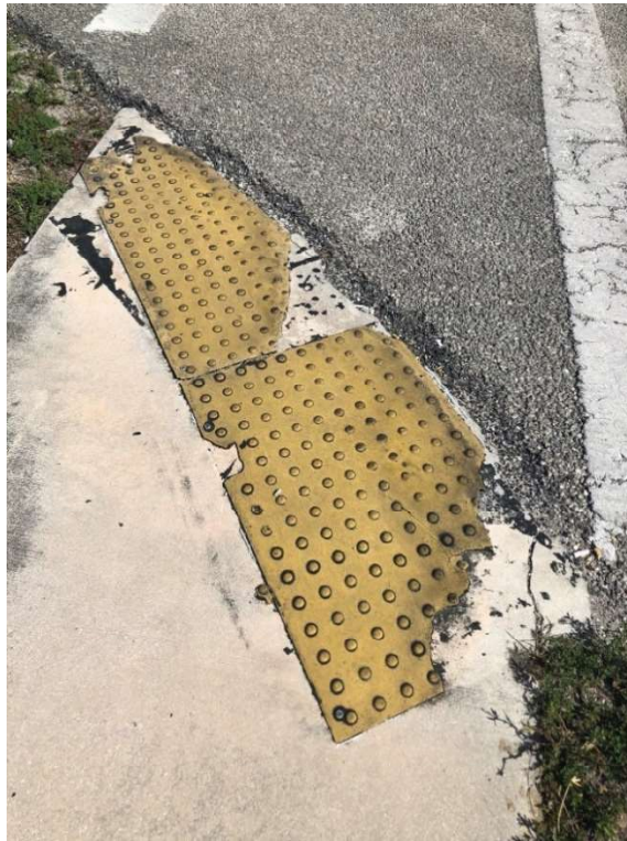
Figure 3: Damaged Detectable Warning Location
