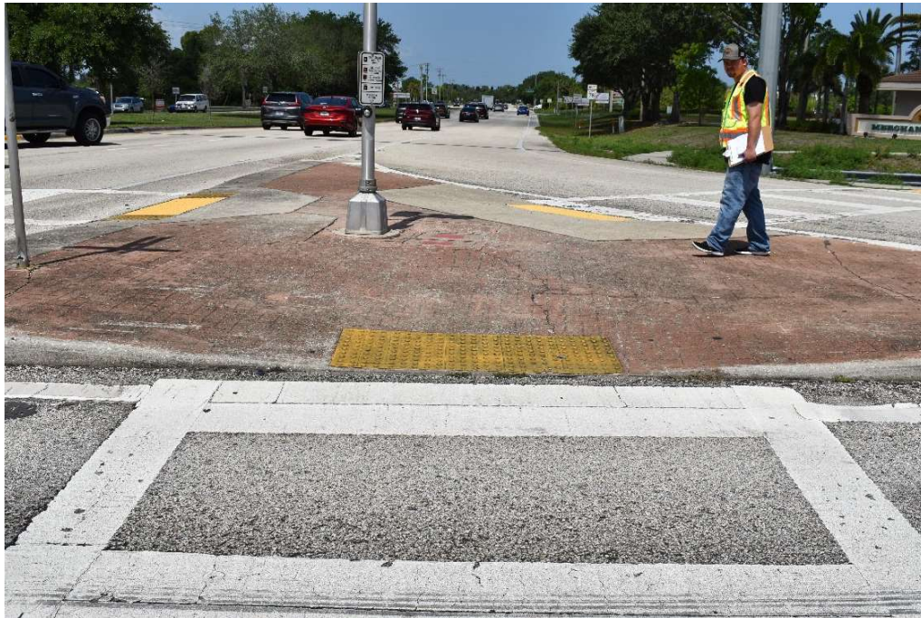
Figure 5: Uncontrolled Crossing at SR 78 (Pine Island Road)
