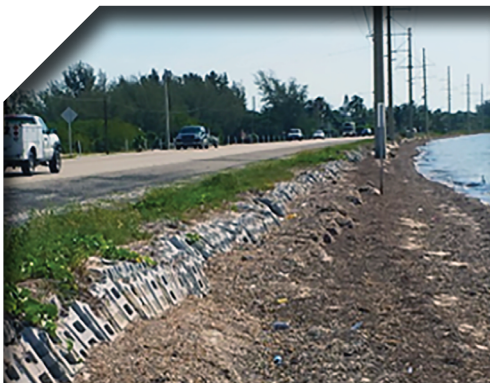
US1/Overseas Highway shoreline protection and road raising near Sea Oats Beach in Islamorada
