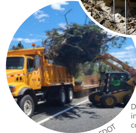
Hurricane Matthew Impact on St. Augustine Beach Source: FDOT
