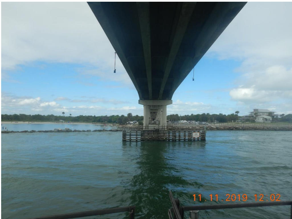
Underdeck of Sebastian Inlet Bridge, facing north along bridge alignment at inlet channel.
