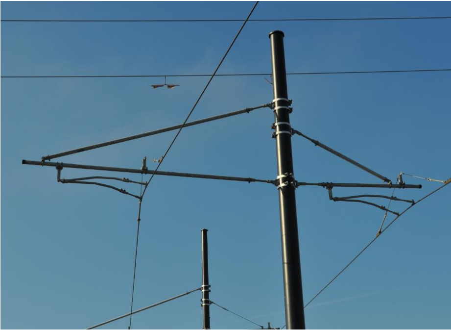
OCS Cantilever with Pole
