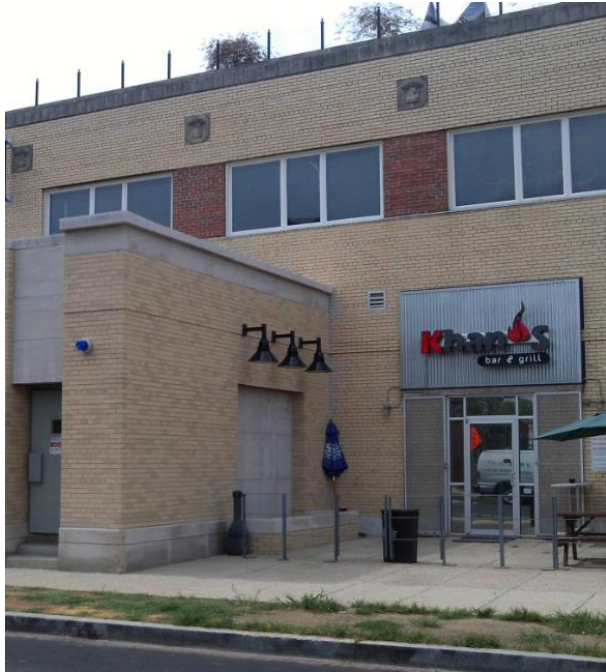
TPSS Integrated within Public Space
