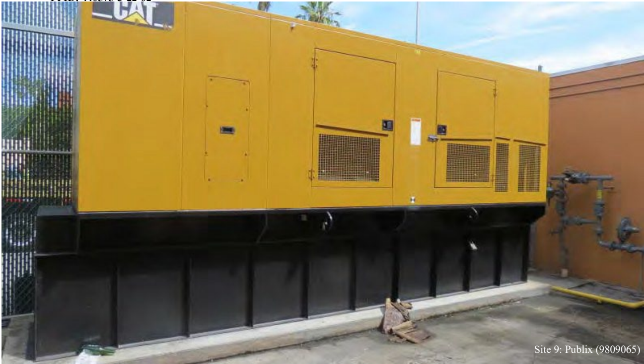
Photo 13. Facing North at Site 9. Below generator AST well maintained, no visible spillage or staining. While front of Publix is 491 feet from existing ROW, the tank is located 711 feet from project. No expected impact to project corridor
