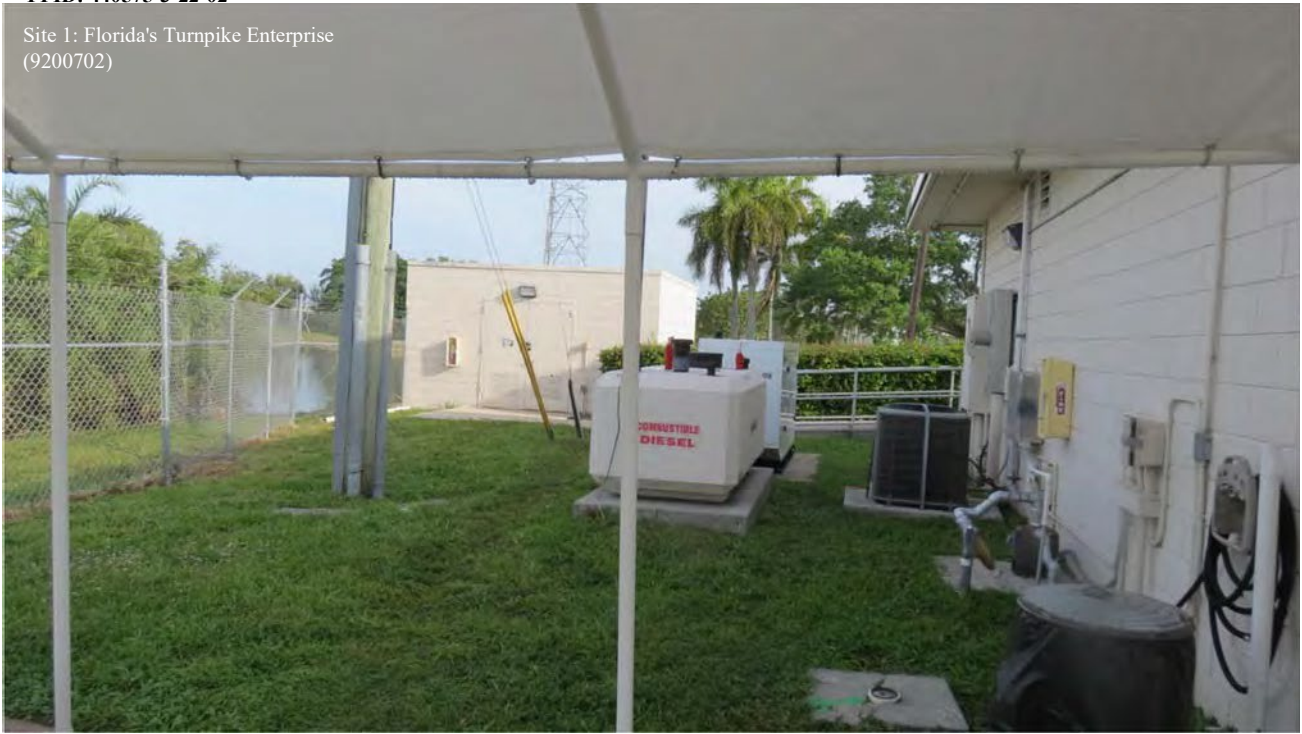
Photo 1: Facing North from picnic area. Located north of the project corridor. AST at Delray Beach FTE Toll plaza. Stormwater pond visible to left. Tank and Generator well maintained. No potential impact to proposed project.
