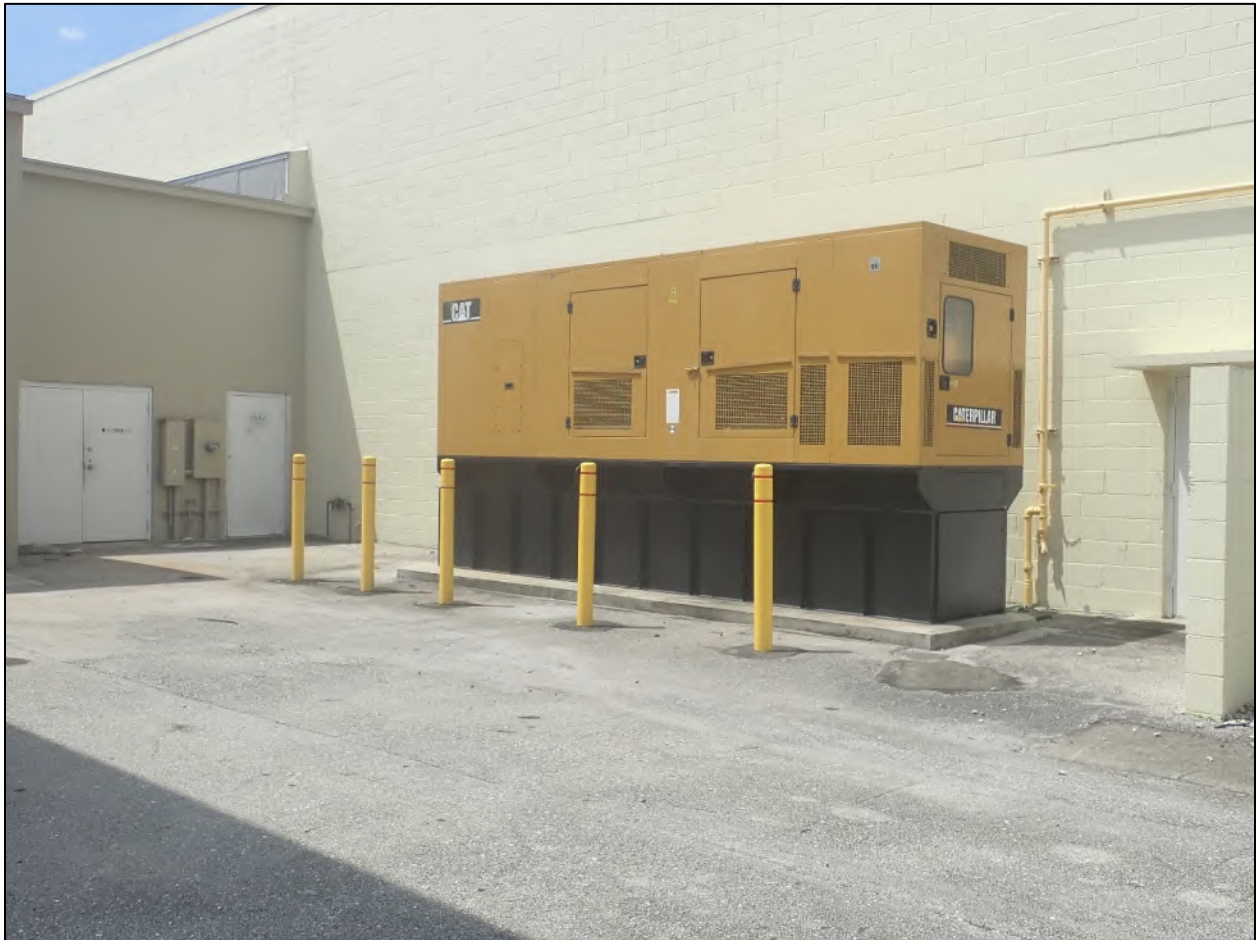
Site # 2 – Publix Food Store Generator
