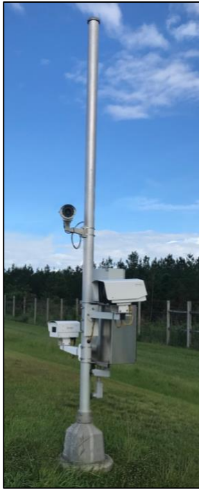
Figure 5. USDOT reader camera and illumination devices.
