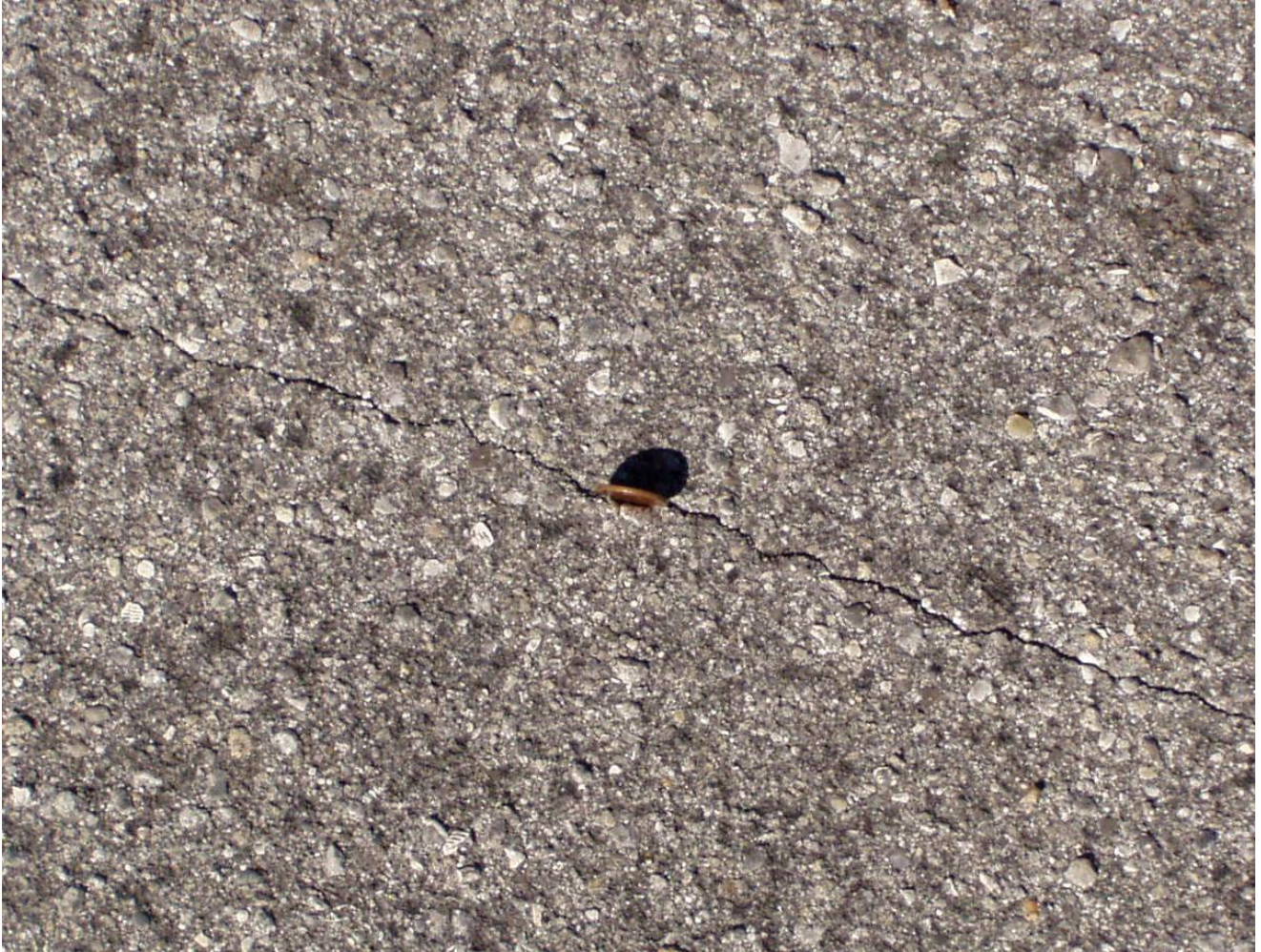
FIGURE 8. CLASS I CRACKING
