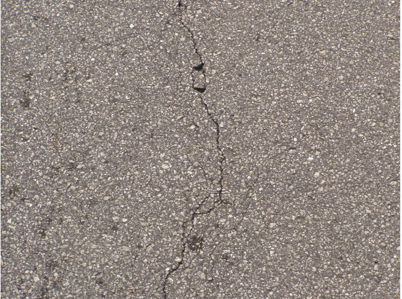
FIGURE 9. CLASS II CRACKING
