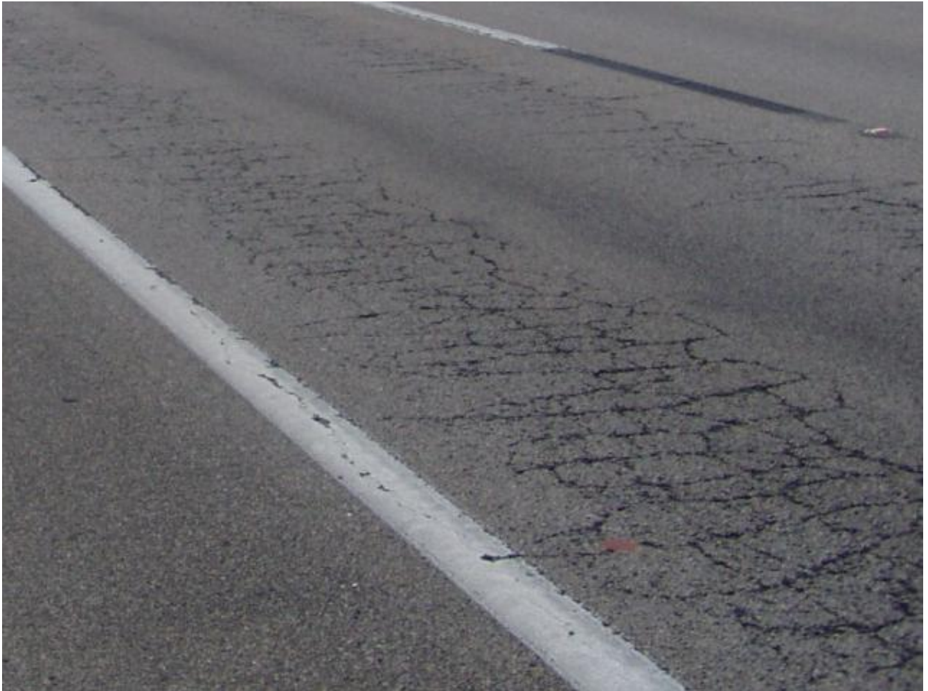
FIGURE 10. CLASS III CRACKING
