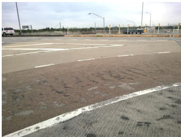
FIGURE 15 – Aggregate loss over concrete.
