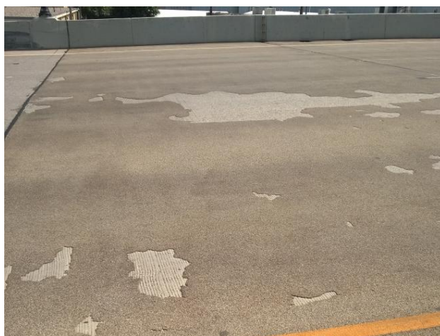
FIGURE 16 – Delamination of a bridge deck overlay.
