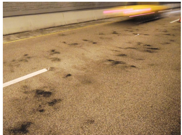
FIGURE 18 – Soft splotchy areas shortly after construction.
