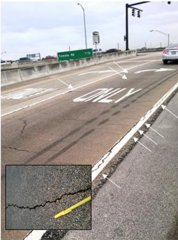
FIGURE 21 – Substrate top-down tearing at a signalized approach (transverse cracking).
