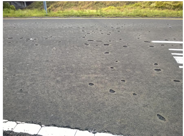
FIGURE 17 – Widespread localized failures due to poor binder mixing.
