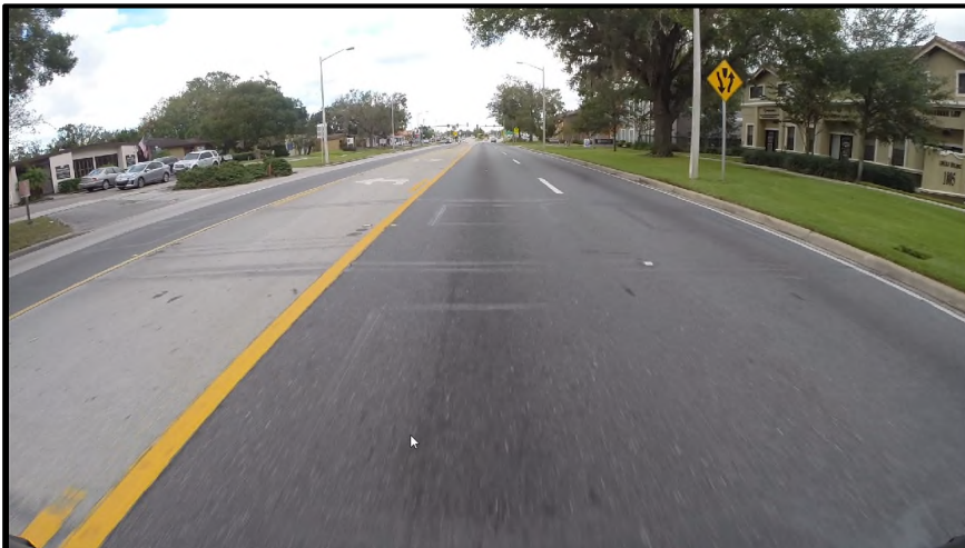
MP 15.475 Westbound – Another view of the maintenance resurface patch on westbound travel lanes as done under maintenance contract #E5Q88. The traffic count loops are embedded in the pavement surface and it is for Count Station #5180.
