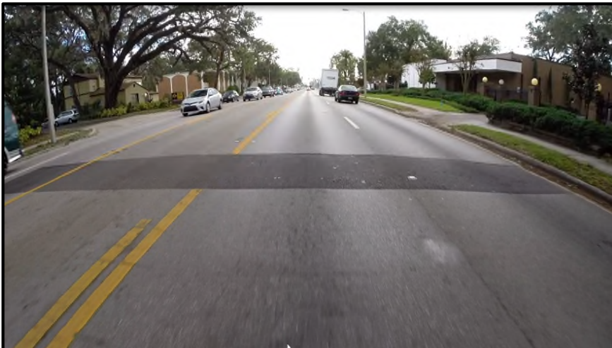
MP 15.750 Eastbound – A view of the trench pavement repair patch for a lateral sanitary sewer repair connection from the main sewer “trunk” line to the clean-out point (just outside of the sidewalk on south side).
