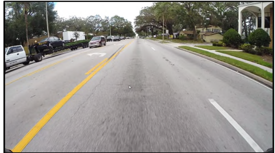
MP 15.814 Westbound – A view of minor branch/longitudinal cracks on the inside (L1) travel lane. Based on MPSV data, this roadway is exhibiting a parabolic cross slope typical section.
