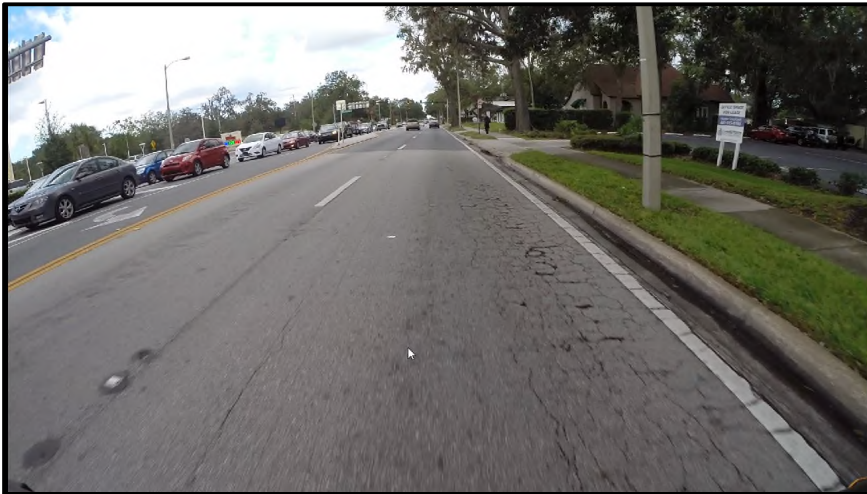
MP 15.932 Westbound – A view of the severe alligator cracks in the right wheel path of the outside (L2) travel lane. Some moderately spalled interconnected cracks creating mini-potholes/voids. The darker pavement surface up ahead is from recent resurfacing work as part of the Wawa permit project – new gas station/store.
