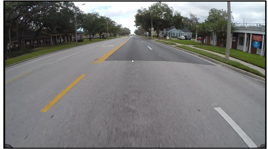
MP 15.670 Westbound – A view of 1,530-ft long maintenance resurface patch in both (L1/L2) travel lanes. This repair work was done in 2013 to address the severe rutting that was occurring in the travel lanes at the time. It was milled 1.5” deep and resurfaced with 1.5” of FC-12.5 friction course.
