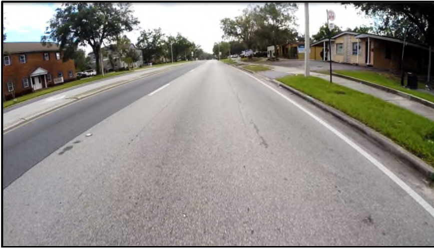
MP 15.386 Eastbound – A view of the 16-ft wide outside (R2) travel lane. Core #4 revealed a split pavement composition as it is apparent there was some pavement widening from the Tampa Avenue intersection (SE quadrant). Also, there is a 575-ft long maintenance resurface patch on the inside (R1) travel lane.
