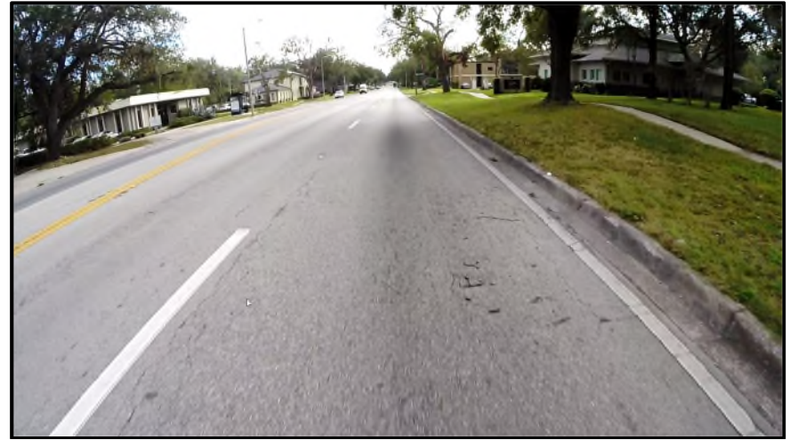
MP 15.506 Eastbound – On the right wheel path area of the outside (R2) travel lane, there is some branch/early stage alligator cracking at this location. Pavement rutting is minor and it is not as severe as seen in westbound (L2) travel lane.
