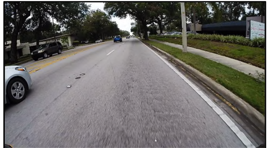
MP 15.722 Westbound – A view of the light to moderate branch cracking on the outside wheel path area of the outside (L2) travel lane. There is some pavement drop-off at the interface with the outside curb & gutter. The drop-off is observed to vary from 0.1 inch to 0.8 inch within the project limits.
