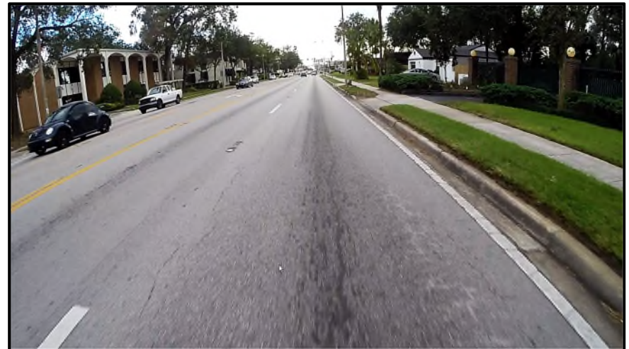
MP 15.780 Eastbound – A view of light limerock pumping in the branch/alligator cracks. The crack severity is light and not significantly extensive. This condition is expected to worsen over time.
