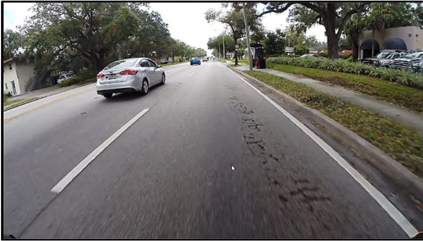
MP 15.704 Westbound – A view of the severe alligator cracks occurring in right wheel path of the outside (L2) travel lane. According to the MPSV data, pavement rutting is prevalent on this lane more so than in any other travel lanes. Note the numerous pop-outs of asphalt material in the wheel path areas.
