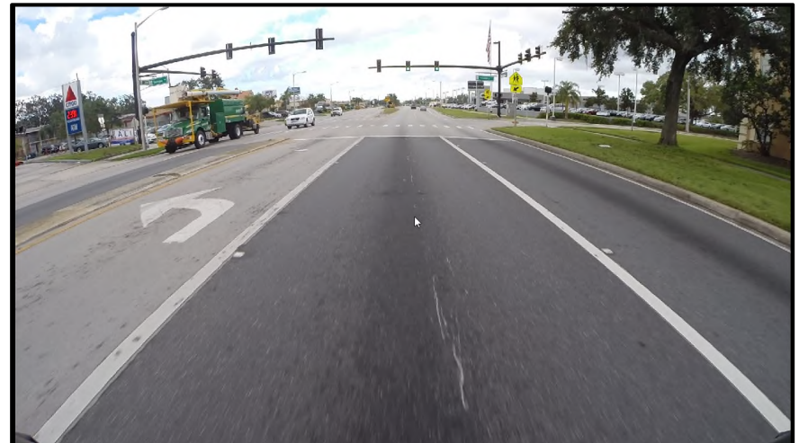
MP 15.398 Westbound – A view of the maintenance patch ending just before Tampa Ave./Country Lane intersection. The center left turn lane with a concrete traffic separator is for SR 50 westbound traffic heading south on Tampa Avenue.
