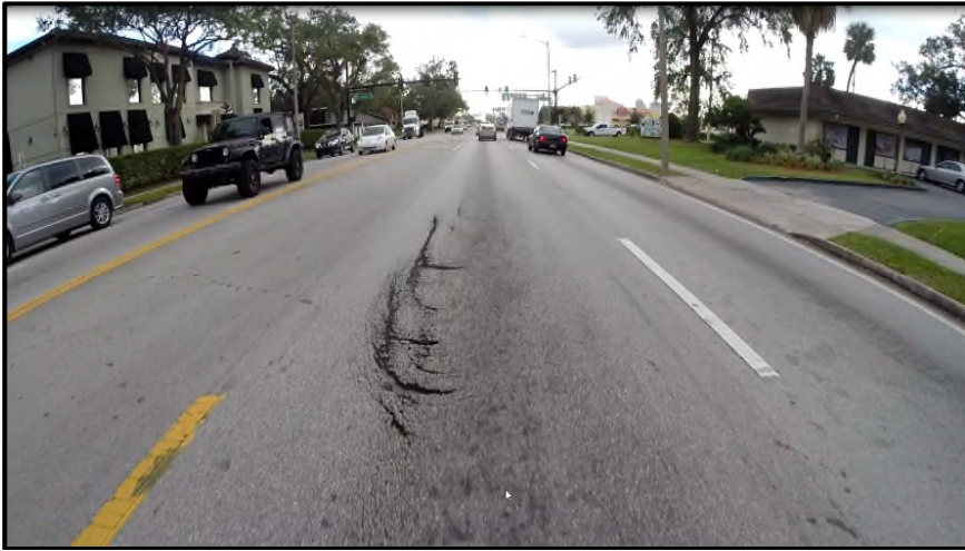
MP 15.820 Eastbound – A view of severe pavement shoving/slippage in the left wheel path of the inside (R1) travel lane. The last mill/resurface project only milled 1” deep and resurfaced 1” FC-9.5 friction course.
