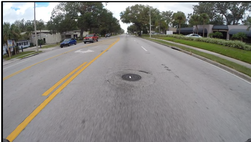
MP 15.737 Westbound – A view of the sanitary sewer manhole structure in middle of the inside (L1) travel lane. Based on review of the GoPro video of this travel lane, there are eight of these type of manhole structures. Note the circular reflective cracking around the manhole frame/cover. It is very likely that concrete is used in the riser/collar connection. A note should be added in the plans to alert Contractor to use caution when milling near/around these manhole structures.
