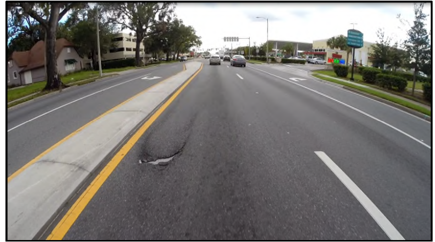
MP 15.880 Eastbound – Another view of pavement shoving/slippage and this is within the area of recently milled/resurfaced work done as a part of the Wawa permit project.
