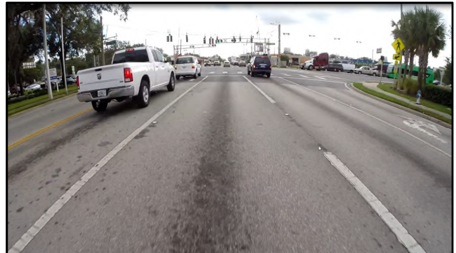
MP 15.940 Eastbound – A general view of the R1 lane as approaching the SR 500/US 441 intersection. Extensive oil drips can be seen in the middle of each travel lane and turn lanes. The project is expected to end at the pavement change joint and not include the entire intersection area.
