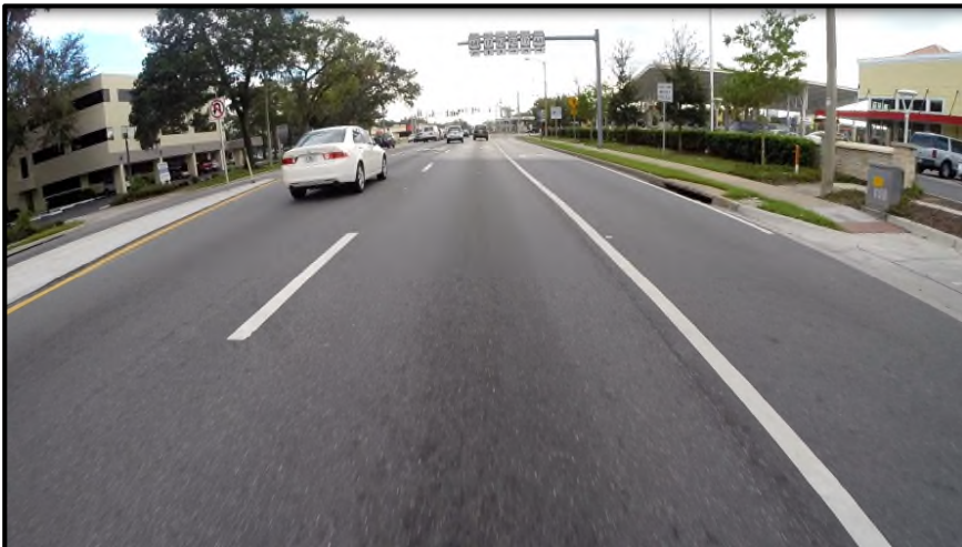
MP 15.902 Eastbound – A general view of the R2 lane in vicinity of recently resurfaced pavement from the Wawa permit project. The new Wawa facility is seen on the upper right corner. The right turn lane is noted to have asphalt base instead of limerock.
