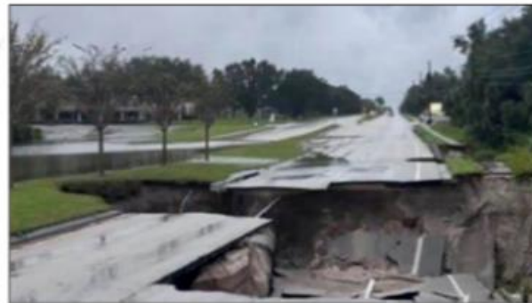
Massive sinkholes were found after Hurricane Milton (example: destruction of infrastructure in Orange City, FL)
