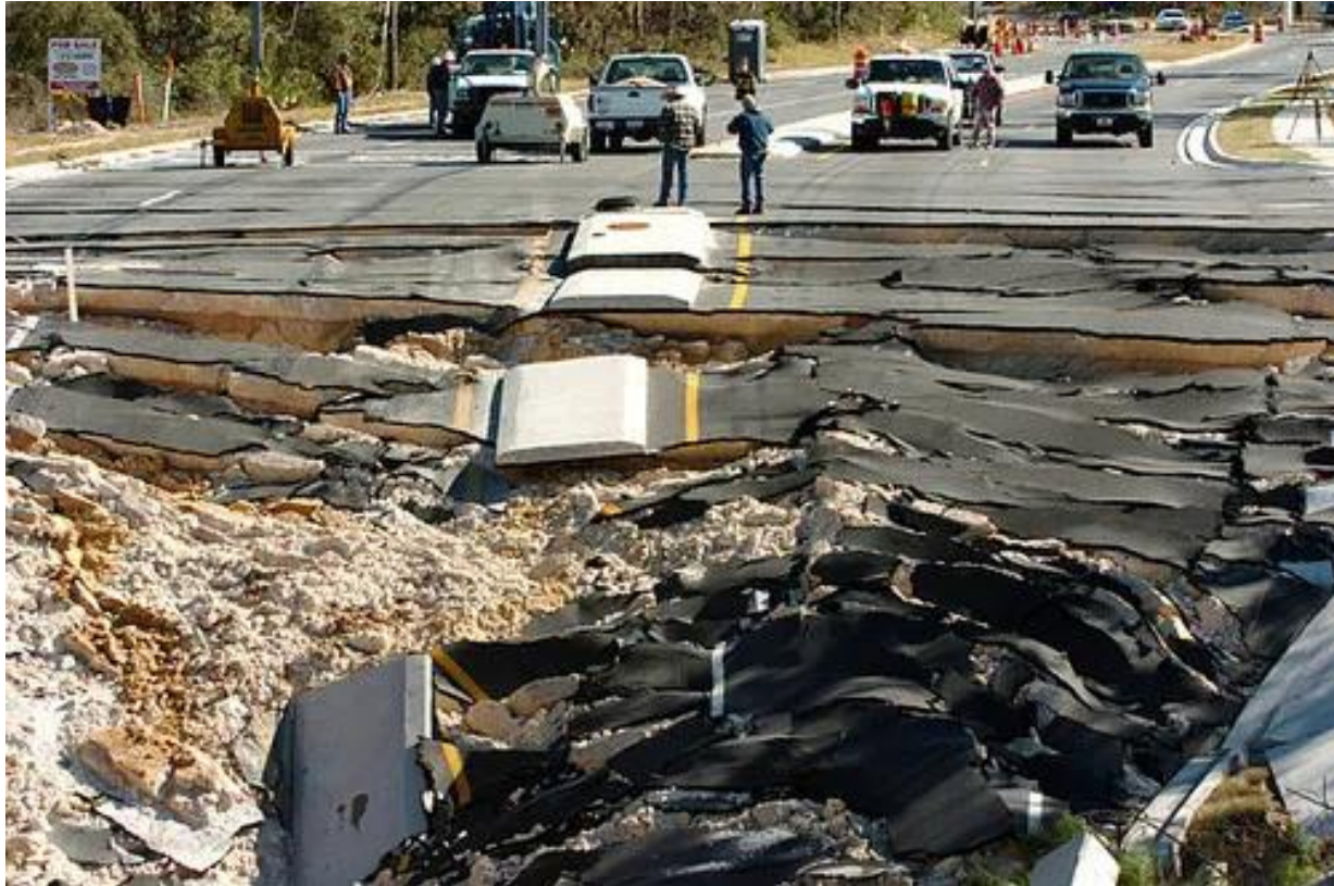
Photo: 2004 Sinkhole Howland Blvd / Barbara Perez, Orlando Sentinel
