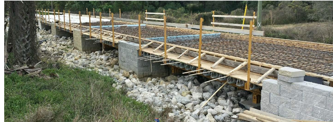
Construction of U.S. 301 Trail Bridge with multi-span GRS-IBS in Zephyrhills, Florida (Danilyarov et al., 2017)
