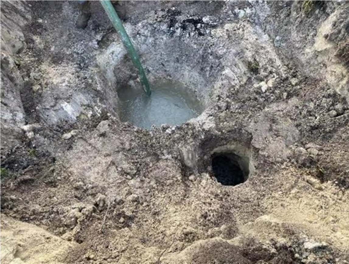
Drill down to 50 ft, Sinkhole shows up
