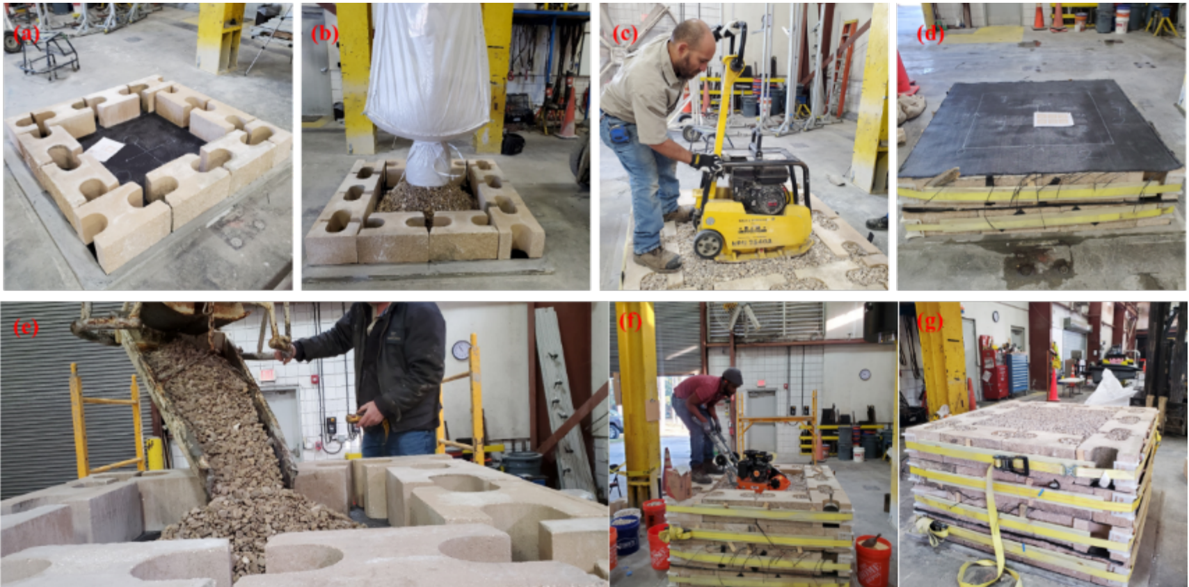
GRS test pier construction steps. (a) Laying the face blocks, (b&c) Placing and compacting backfill, (d) Laying down geosynthetics, (e,f, & g) Repeat A-C until the final height is reached
